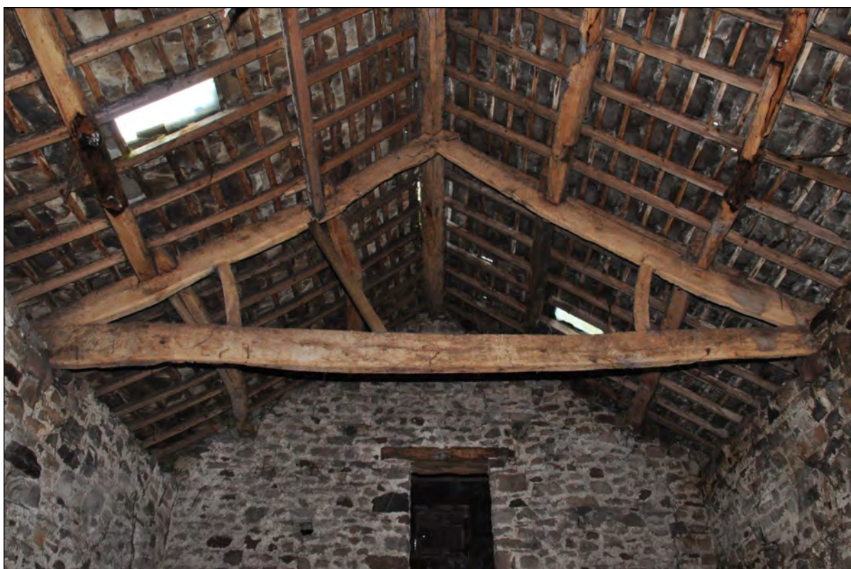
Photo 8: West roof truss. Note that the collar has been removed, and later timbers have been added as repairs.
