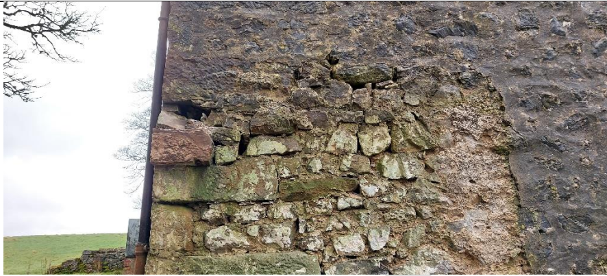
Building B2b (adjoining barn) – west elevation – gaps and cracks in brickwork.
