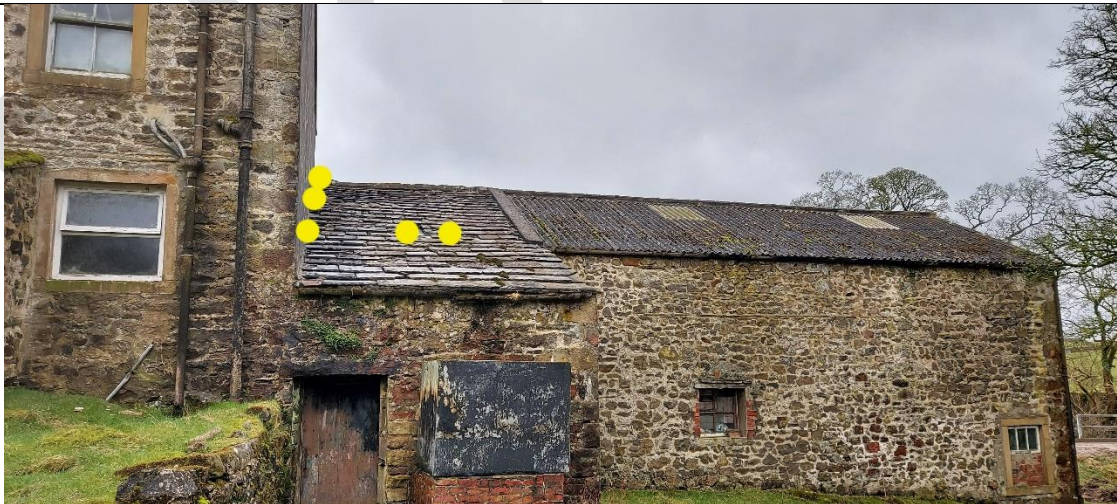
B2a (adjoining barn) – north elevation – gaps under York stone roof tiles.
