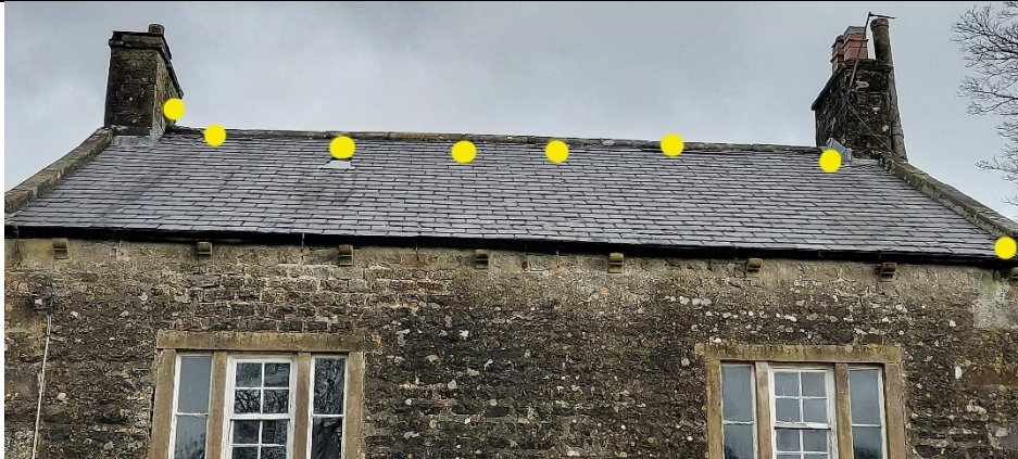
Building B1 (farmhouse) – south elevation (front) - yellow indicates lifted tiles & gaps under flashing.
