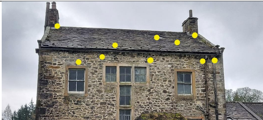
Building B1 – north elevation (rear) - loft interior gaps under York stone tiles, cracks in walls etc.
