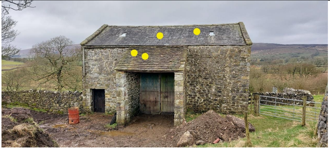
B3 (detached stone barn) – east elevation (front) – highlighting PRF gaps under roof tiles.
