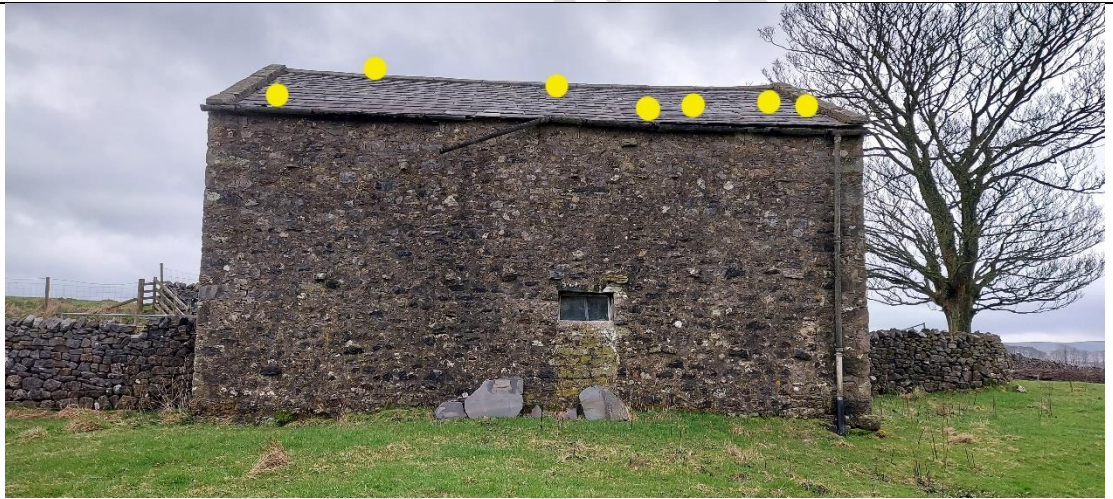
B3 – west elevation (rear) – showing lifted tiles on roof.
