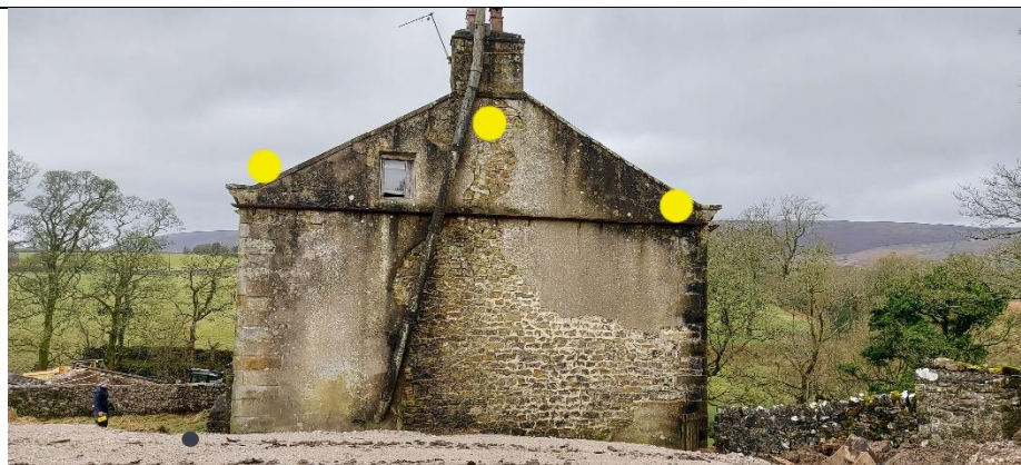
Building B1 – east elevation – gaps and cracks in brickwork
