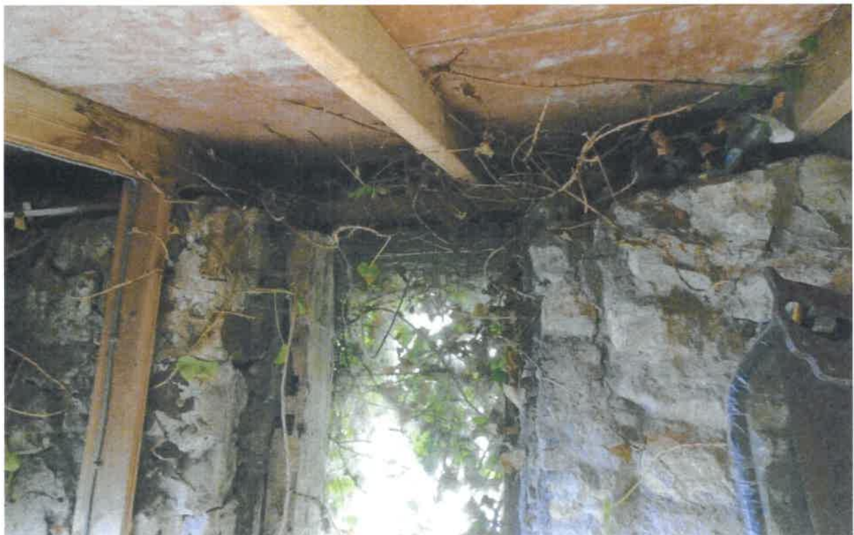
PL07 - Photograph inside the outbuilding, showing the ivy penetration internally.
