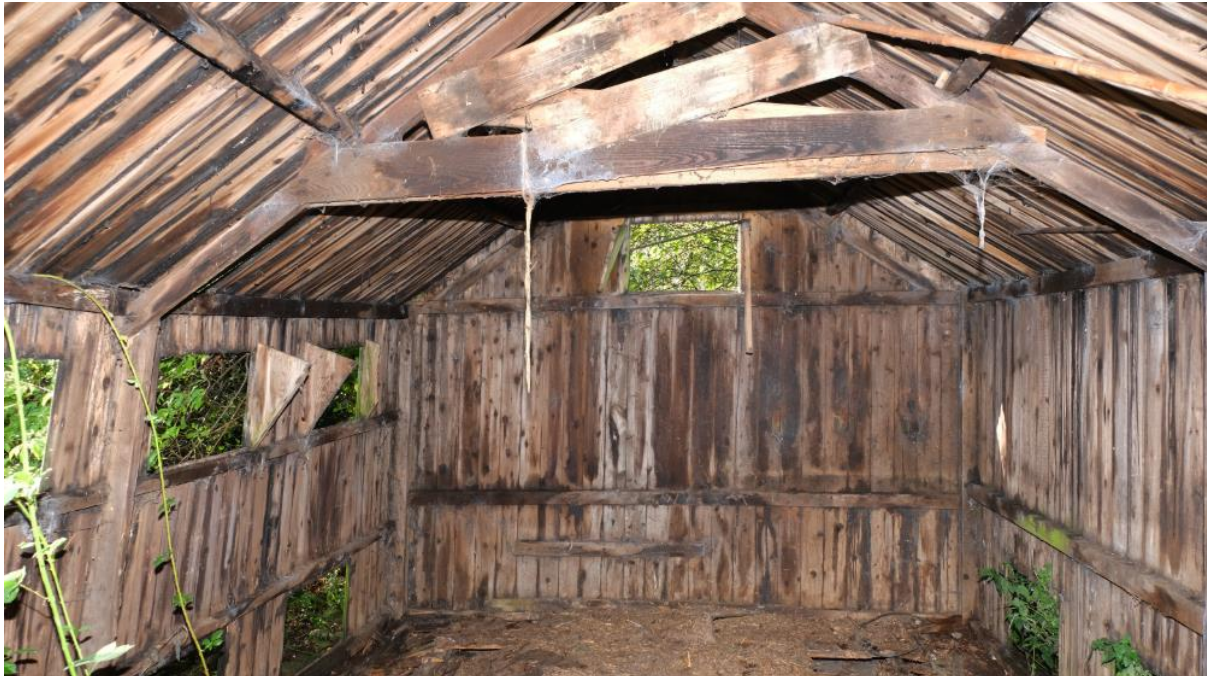
Internal view of one of the timber sheds. Negligible potential for bats but high potential for use by nesting birds.
