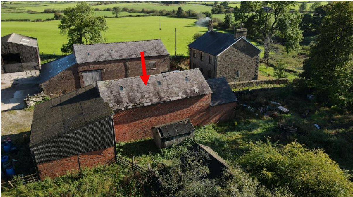
View of the barn building showing slate roof with roof lights, adjoining mono pitch asbestos hay barn (lhs) with areas of unmanaged, disturbed land in the foreground and other farm buildings in background.
