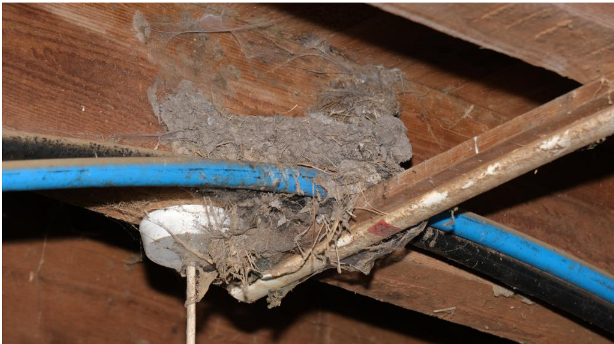
Swallow nest found on the ceiling of the ground floor
