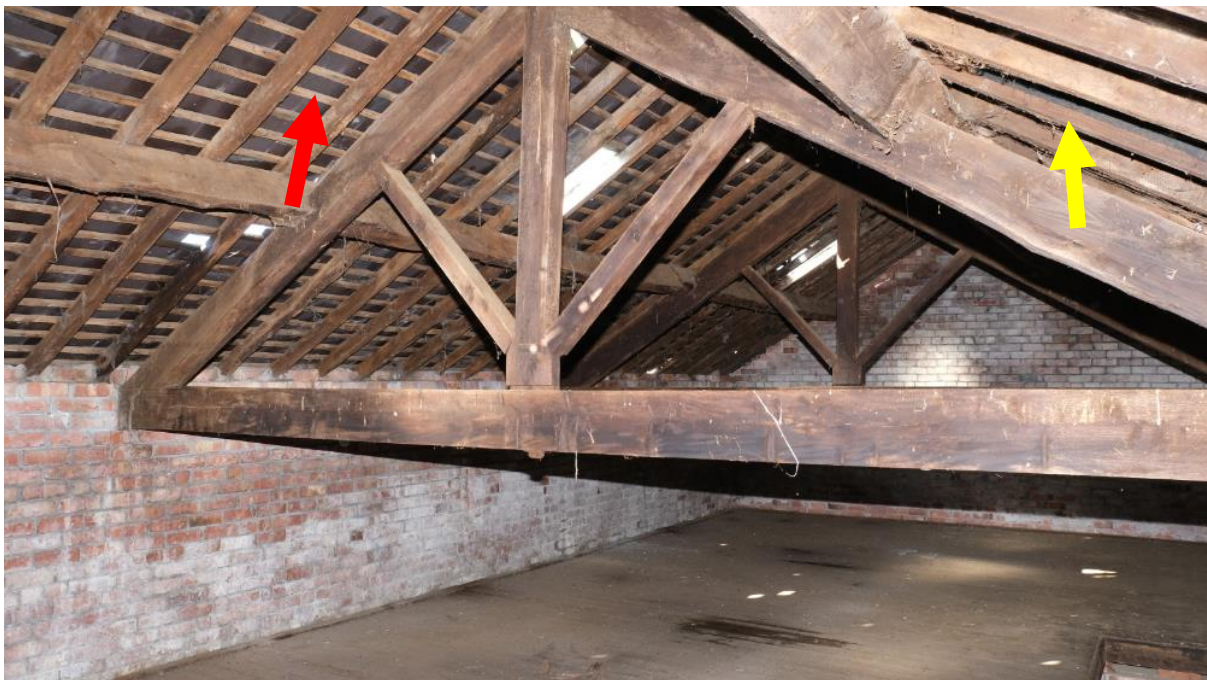
Internal view of the first floor. Image showing unlined roof pitch (red arrow) with holes providing fly in access for use by bats, birds and owl; and lined roof pitch to the north (yellow arrow) providing potential day roosting opportunities for bats.
