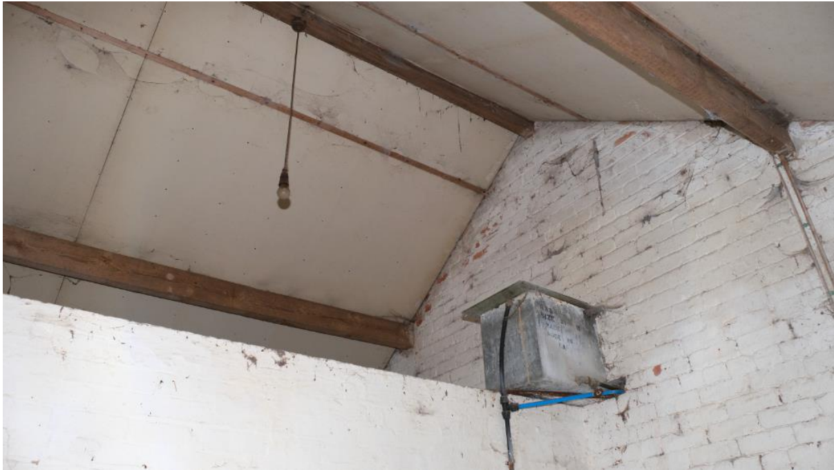
Internal view of the single storey section to the east. Slate roof is underlined with boards providing potential roost feature (gaps between slates and underboarding) for use by bats throughout the year.
