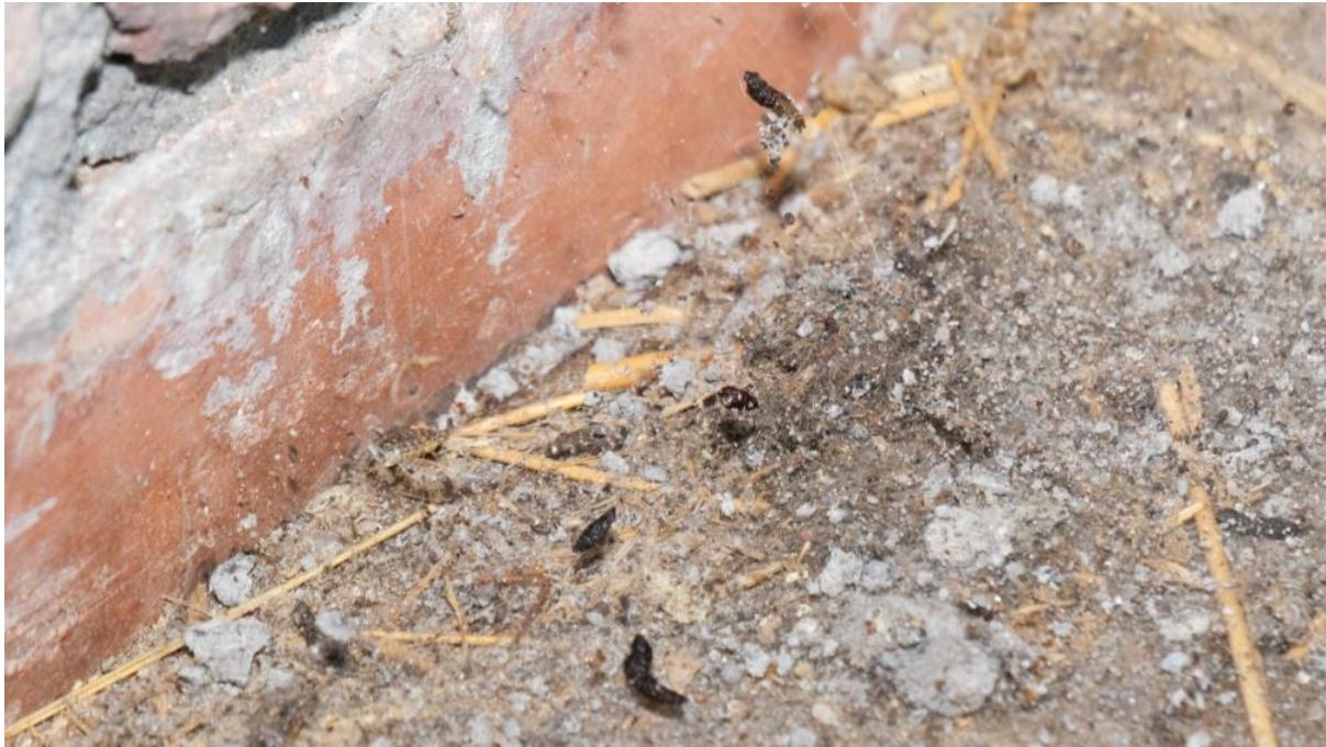
Bat droppings found in the north east corner of the first floor
