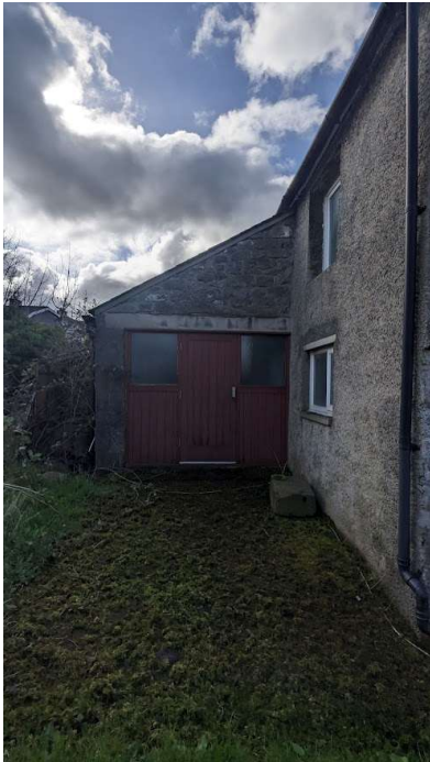
Figure 2 - Picture of Single Storey Garage to the Side and Part of Side Elevation
