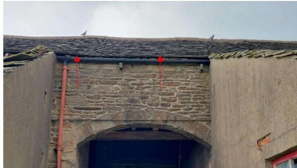
Photograph 6: Southern aspect. Gaps in wall plate.
