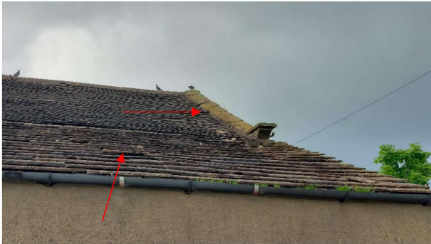
Photograph 5: Southern aspect. Missing mortar on gable end ridge line and lifted tiles throughout.
