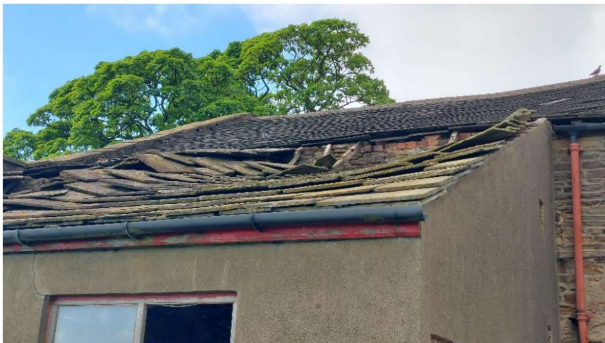
Photograph 7: South western annex. Collapsed roof had created multiple features for roosting bats (likely day roost only in this location).
