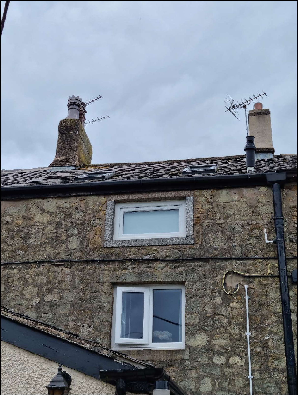
Figure 5 Photograph taken of the roof from the position of the rear extension (source - Jamie Skuse)
