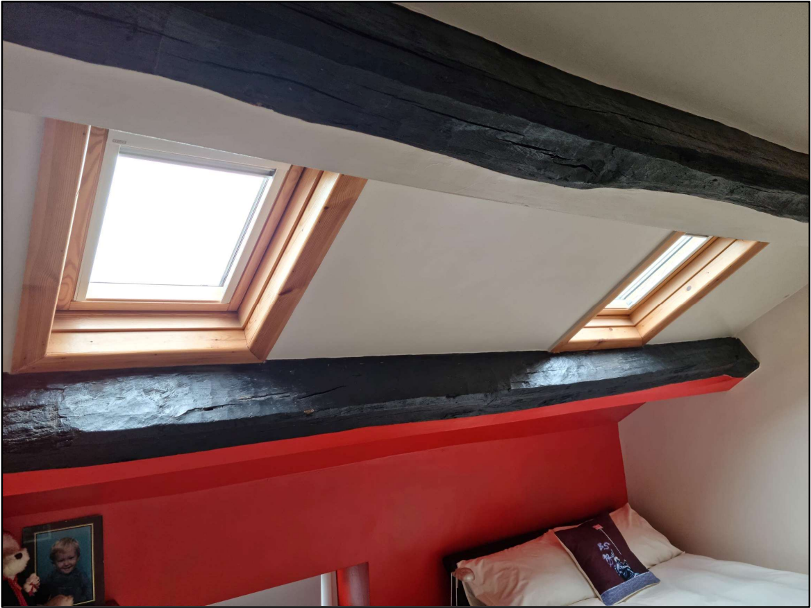
Figure 7 Photograph taken from within the attic looking at the internal view of the rooflights (source - Jamie Skuse)
