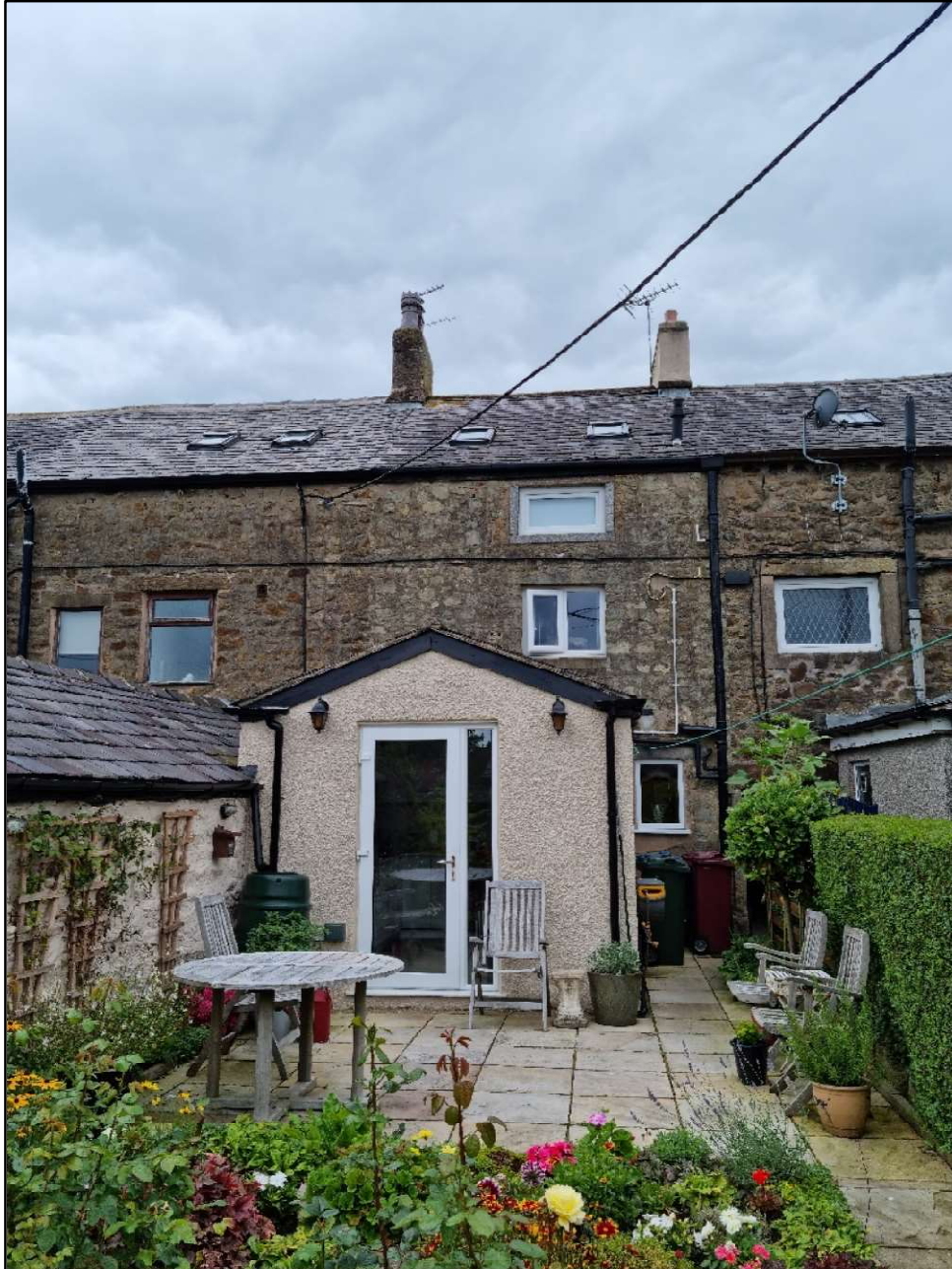
Figure 1 The rear elevation of No 18 Church Street. The two rooflights are located between the two chimneys and are above the attic window at the top of the elevation (source - Jamie Skuse)
