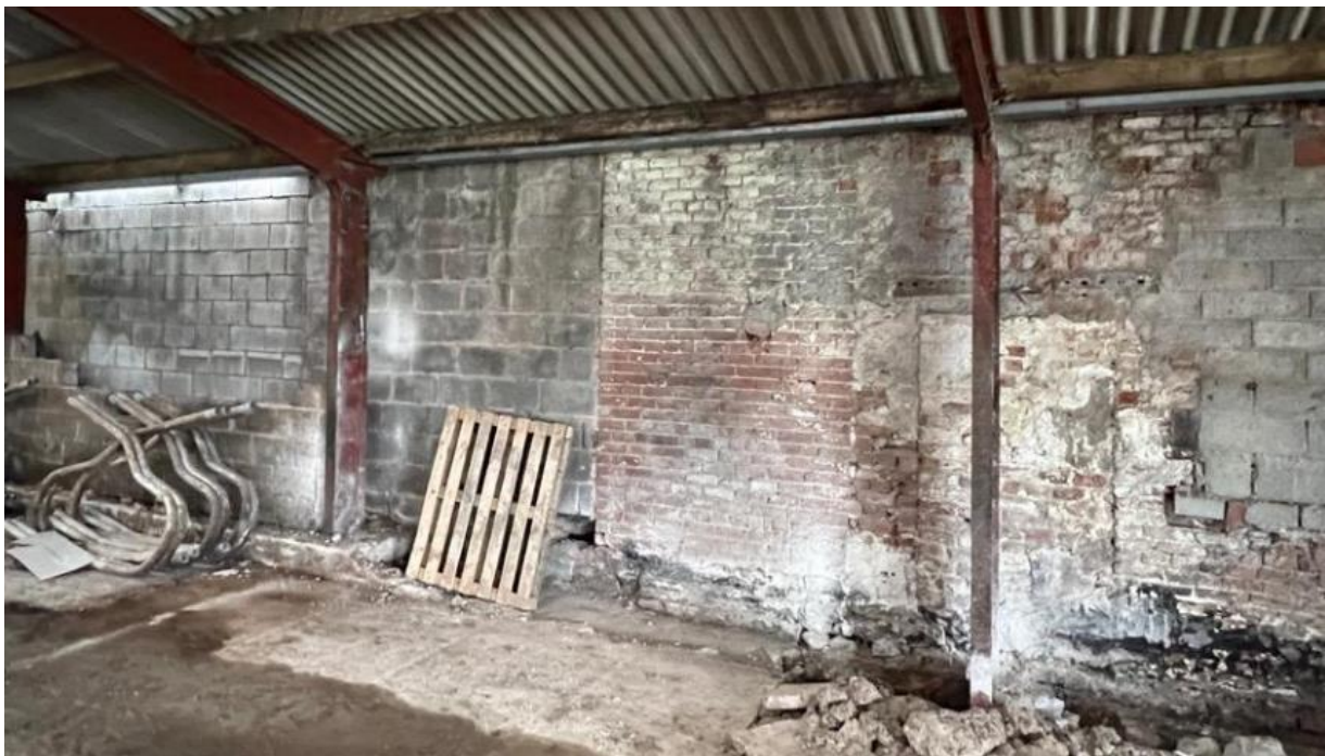
Figure 11) Central portion of southern elevation showing past alterations including blocked door (right) and blocked cart entry (centre left)
