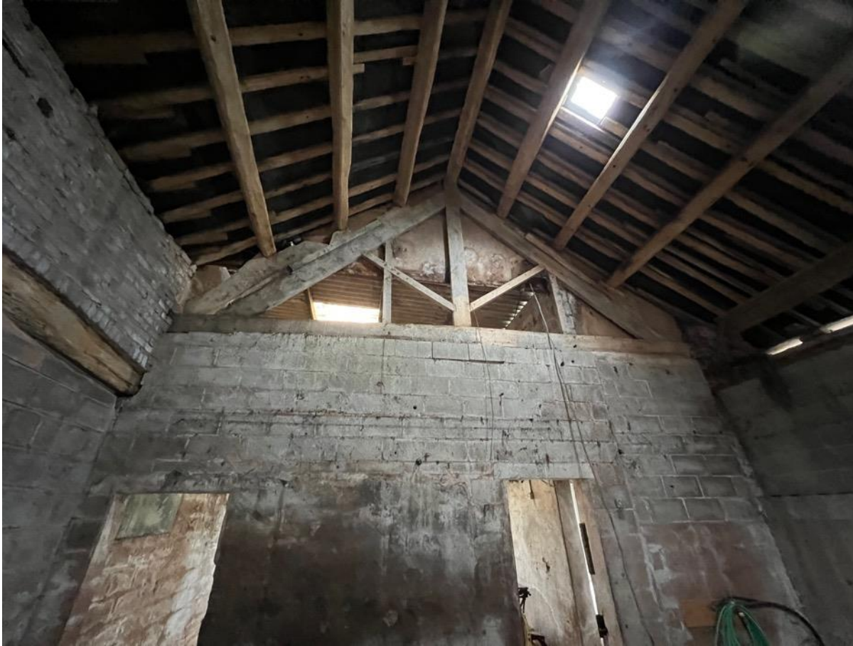
Photo 58 - Internal – main barn – rebuilt gable to main barn to extension at west end
