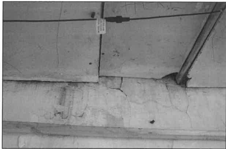
Photo 5: Example of gap in the ceiling boards.
