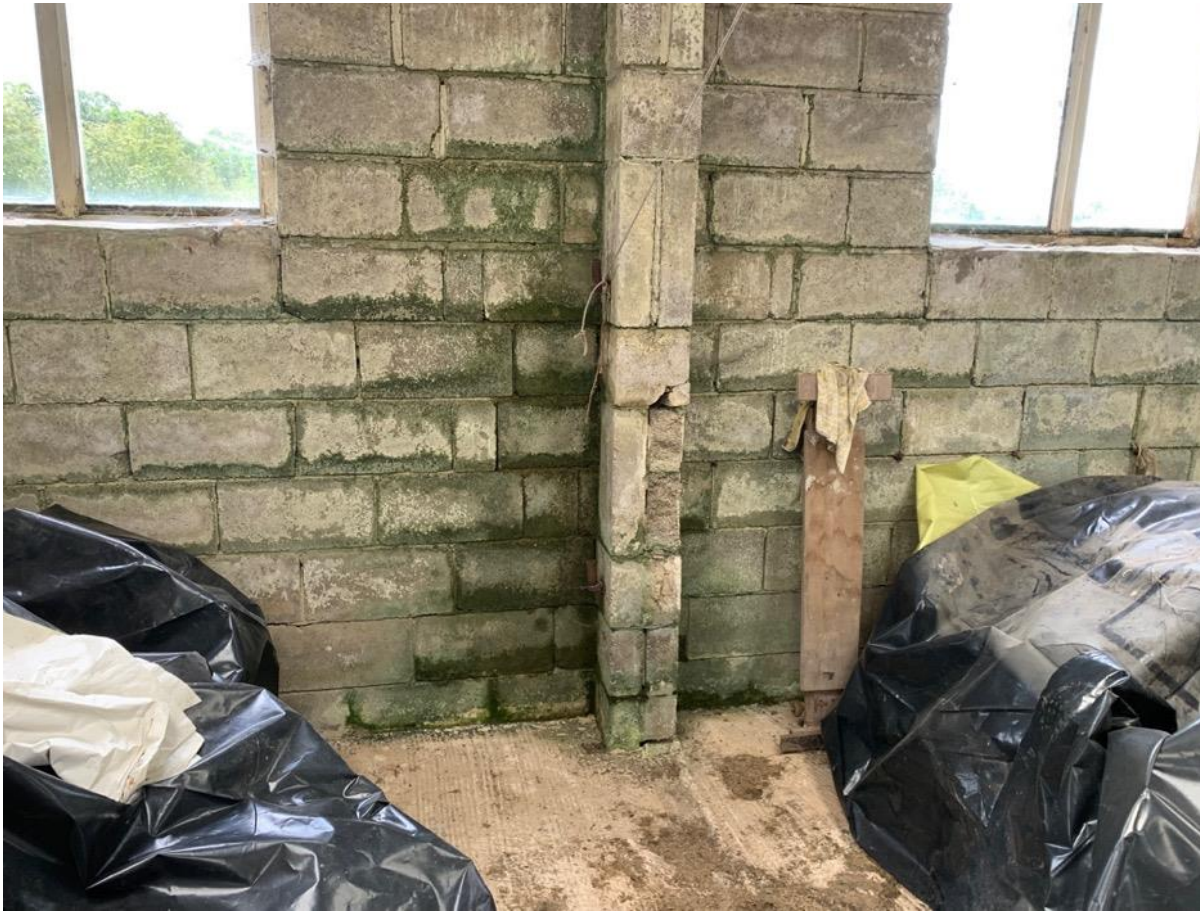
Photo 52 - Internal to newer blockwork building – damp penetration and damage to pier
