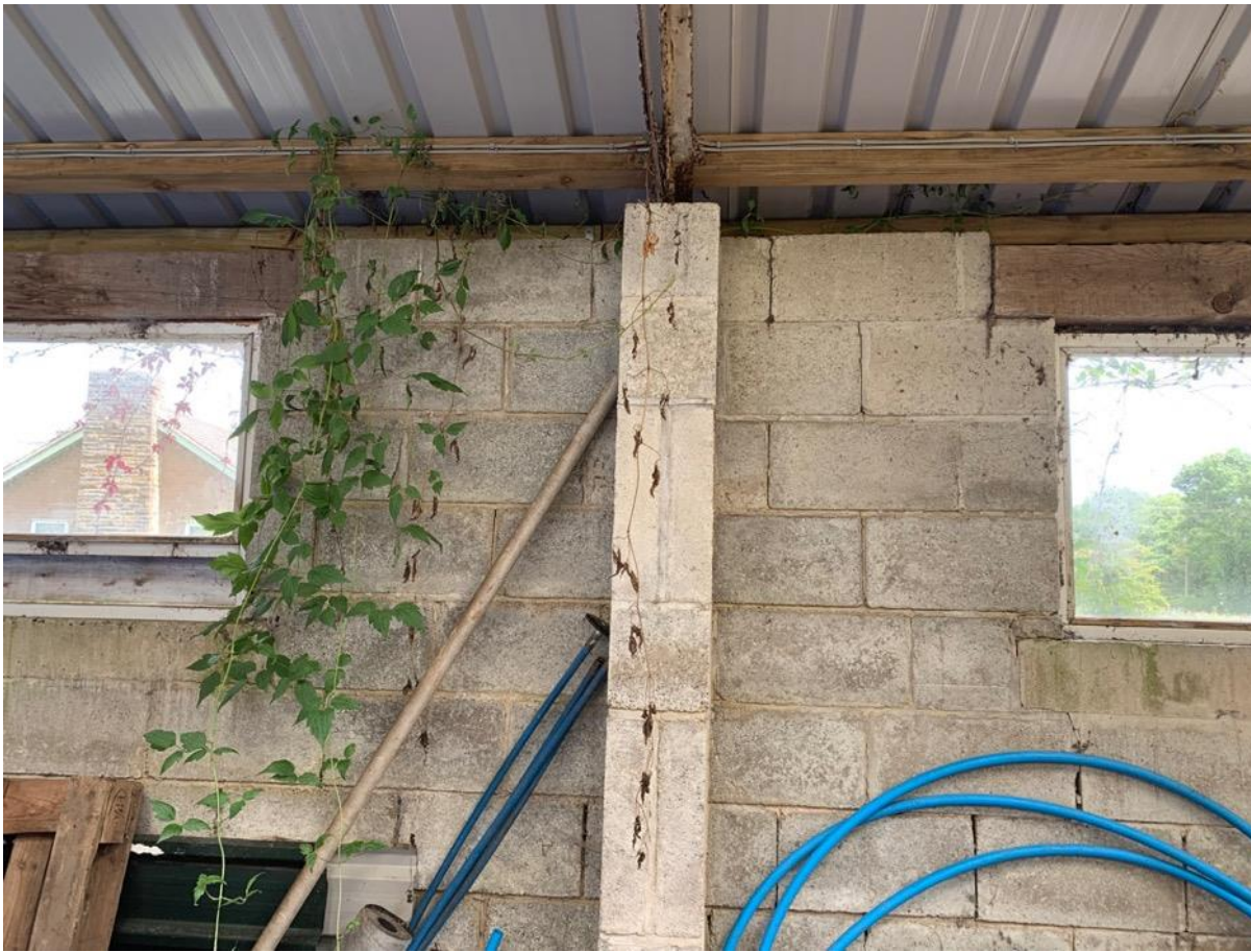
Photo 61 - Internal to newer blockwork building - vegetation
