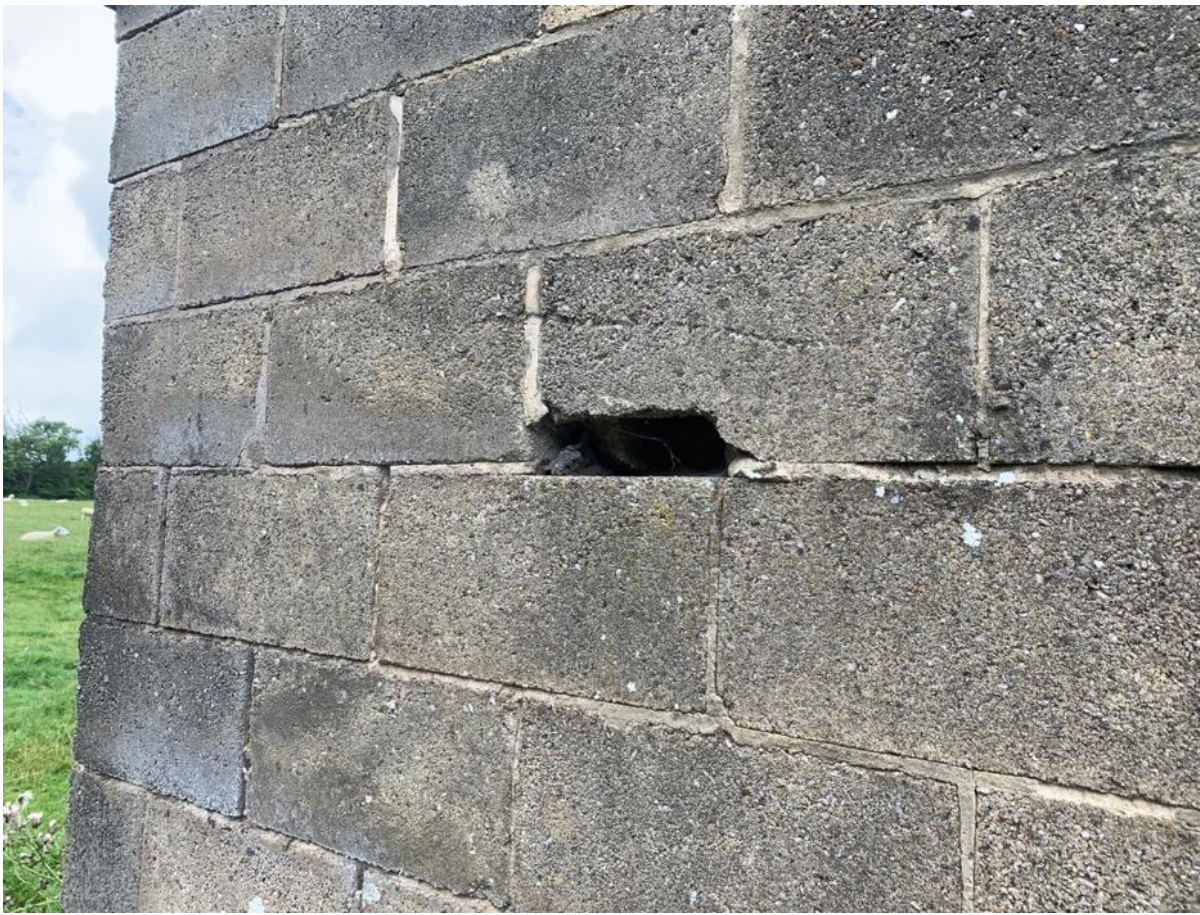
Photo 3 – South Elevation damage
