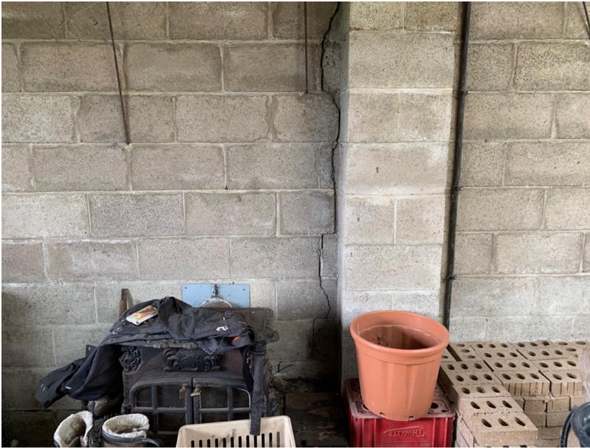
Photo 58 - Internal to original building extension – movement adjacent to pier
