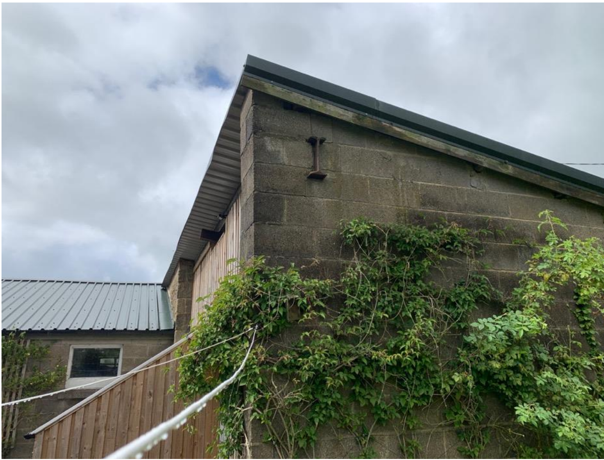
Photo 31 - East elevation of mono-pitch extension to original building indicating sheeting and penetrating I Beam
