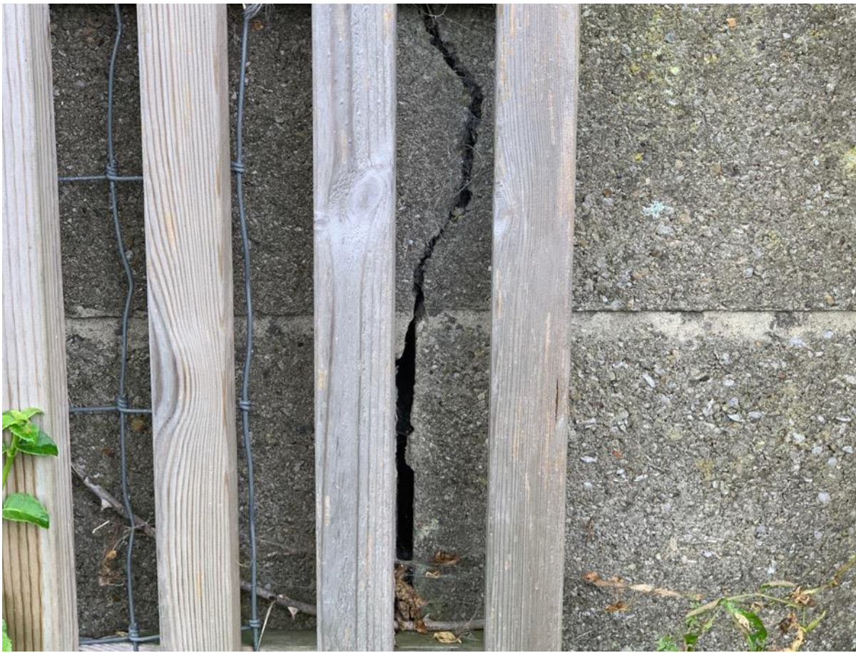
Photo 33 - East Elevation blockwork movement to extension to original building
