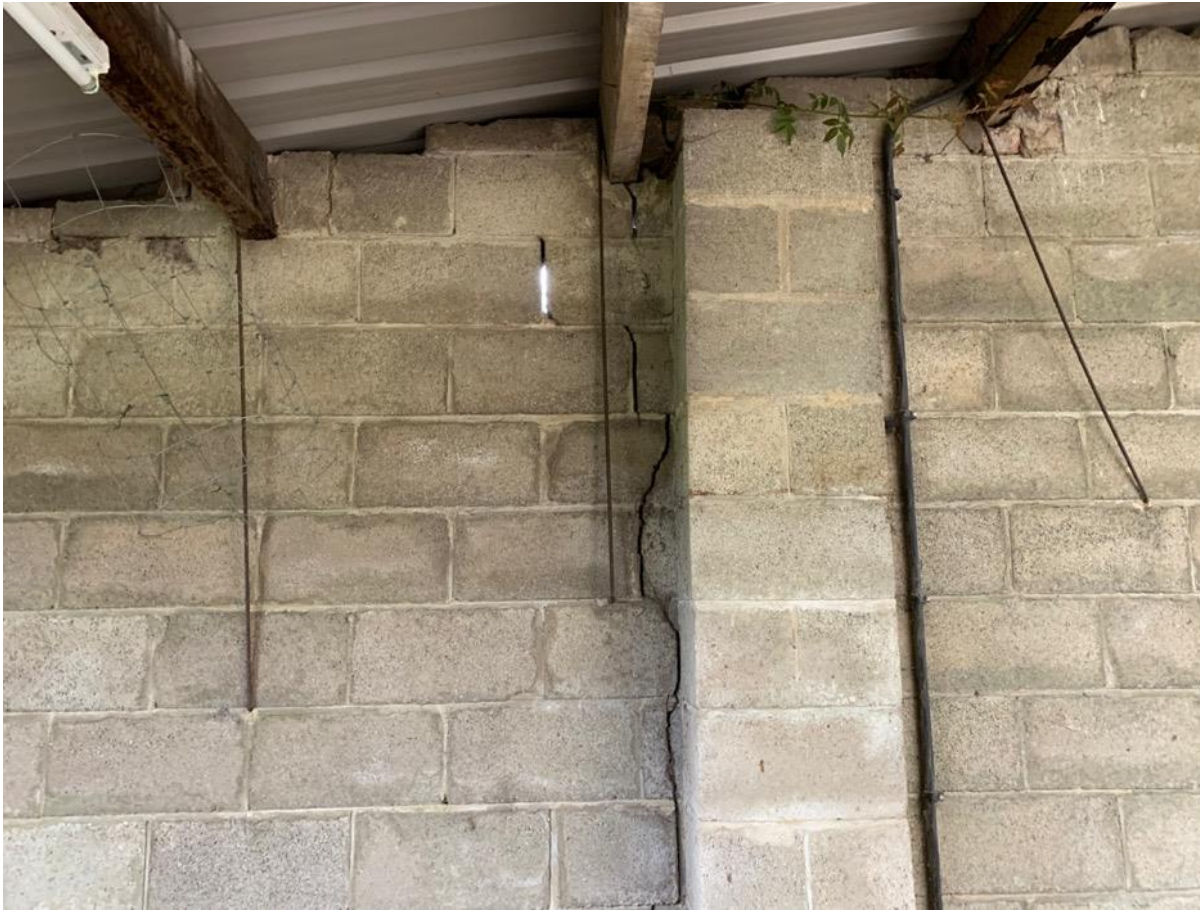
Photo 62 - Internal to original building extension – movement adjacent to pier
