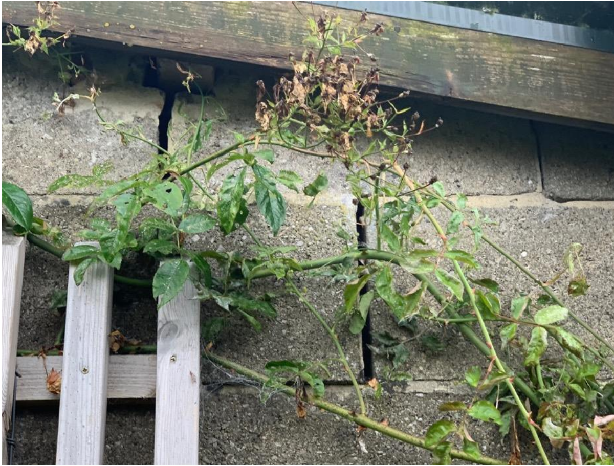
Photo 32 – East Elevation blockwork movement to extension to original building
