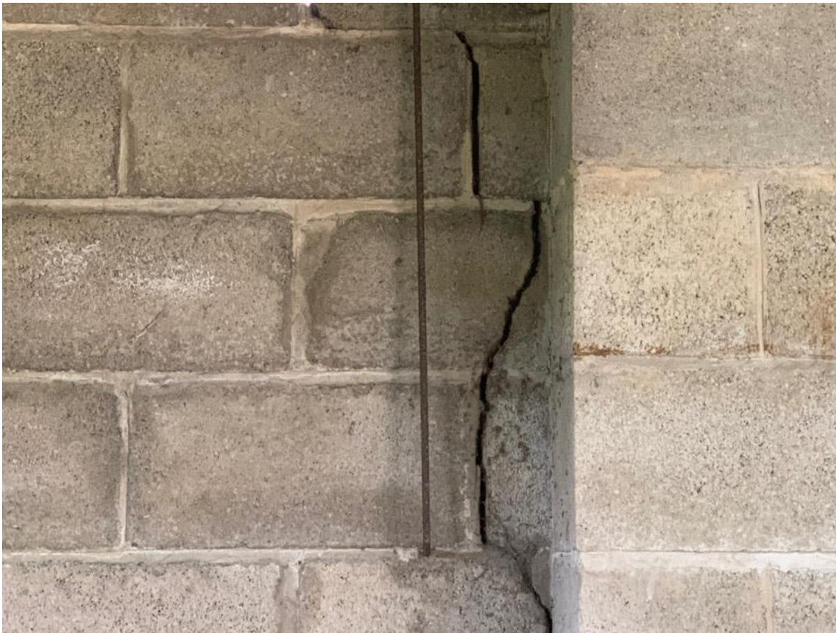
Photo 60 - Internal to original building extension – movement adjacent to pier
