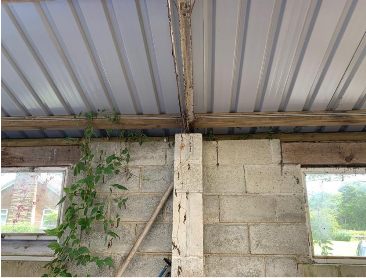
Photo 59 - Internal to newer blockwork building - vegetation
