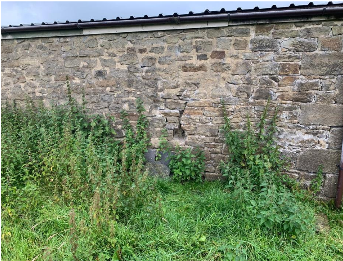
Photo 21 – North Elevation – damage to stone
