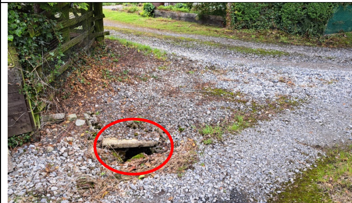
Exposed paving slab with void to the west of the turning head into the adjacent property. A sound of running water could be heard
