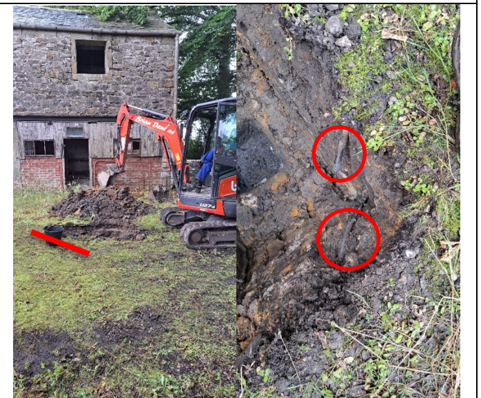
TP2 re-location – in front of barn Black pipe in corner of TP2. Red circles denote pipe and red line denotes route
