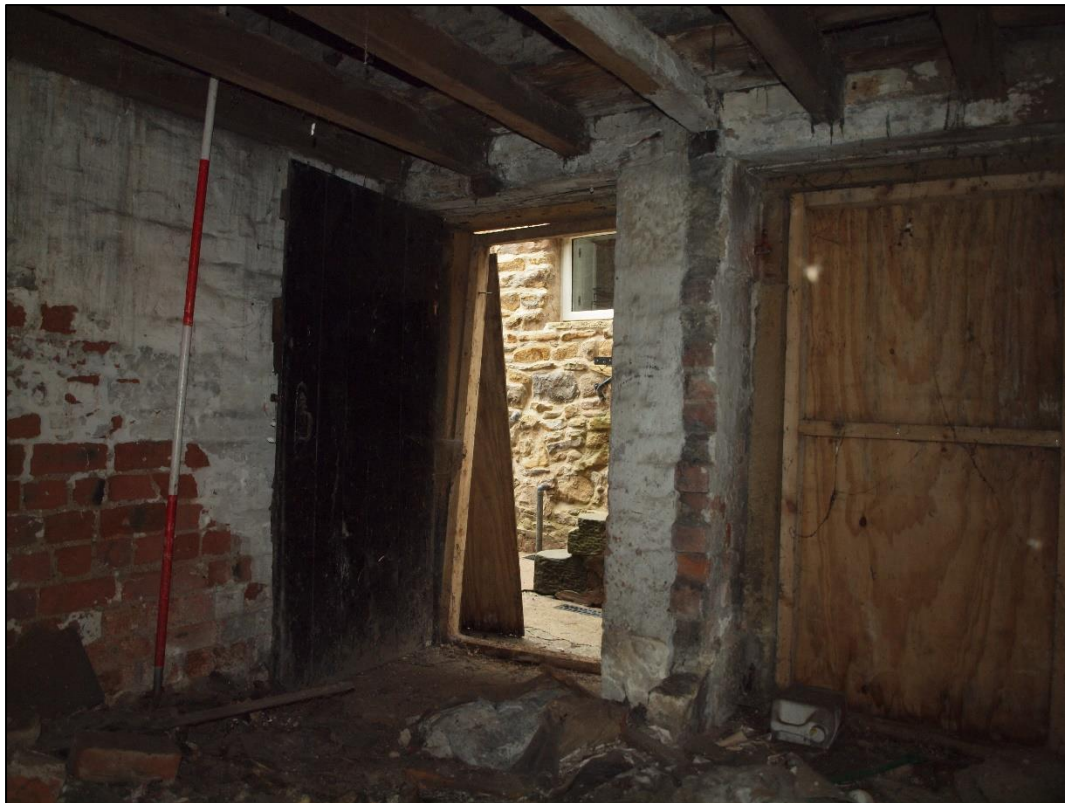
Plate 77: Doorways to west gable showing scar of removed brick wall
