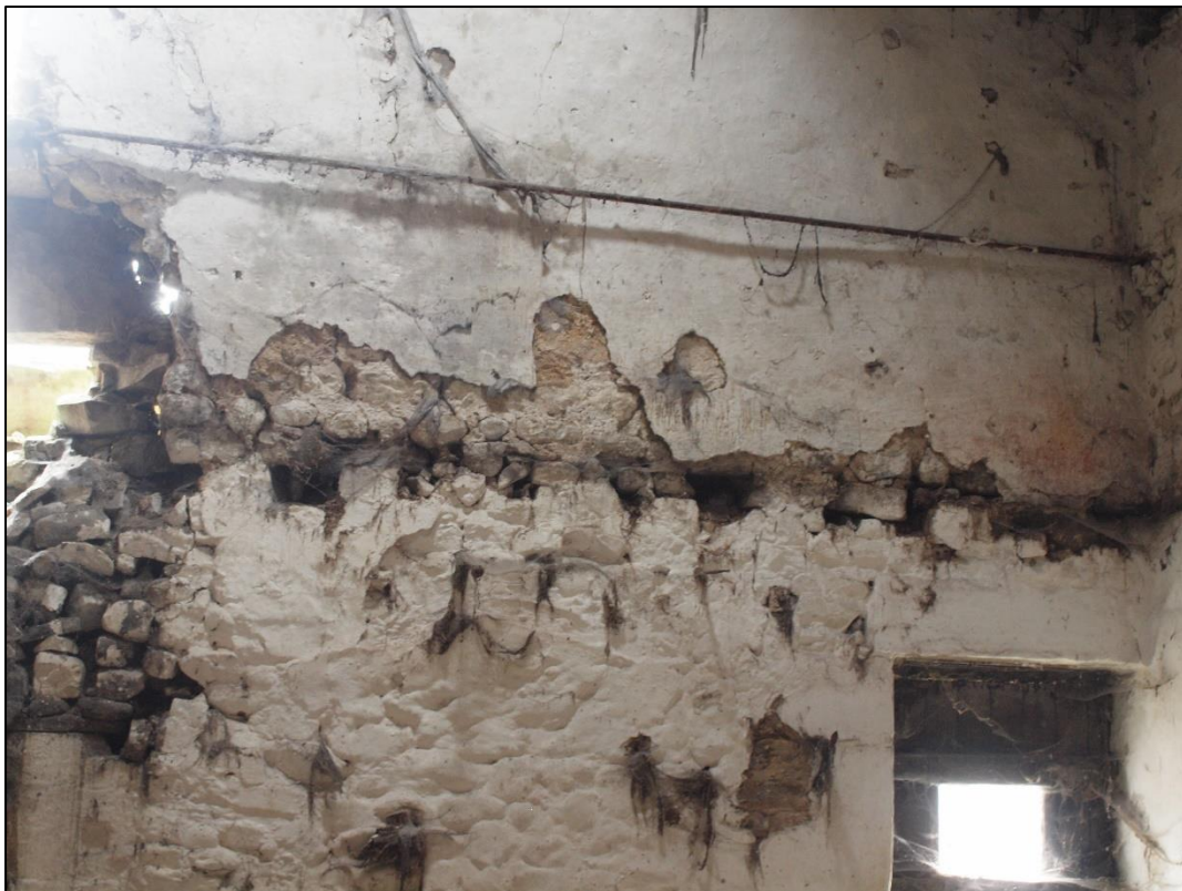
Plate 62: Joist holes in eastern gable
