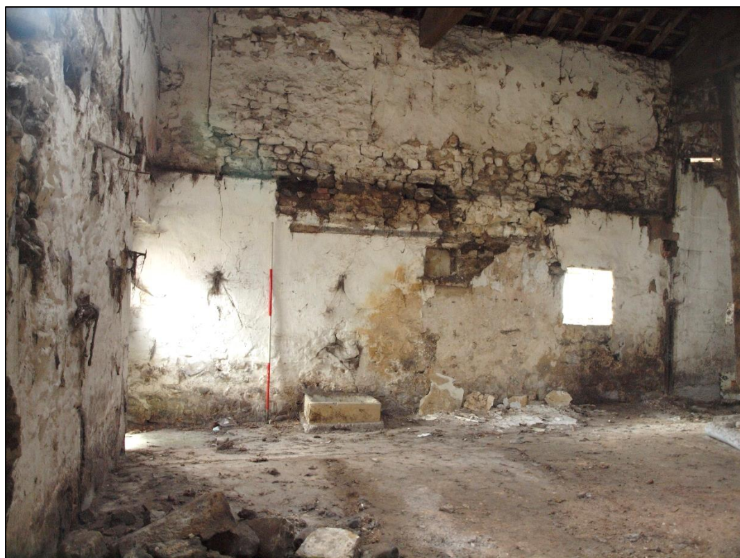
Plate 46: Eastern end of south wall showing blocked first floor window and ground floor niche
