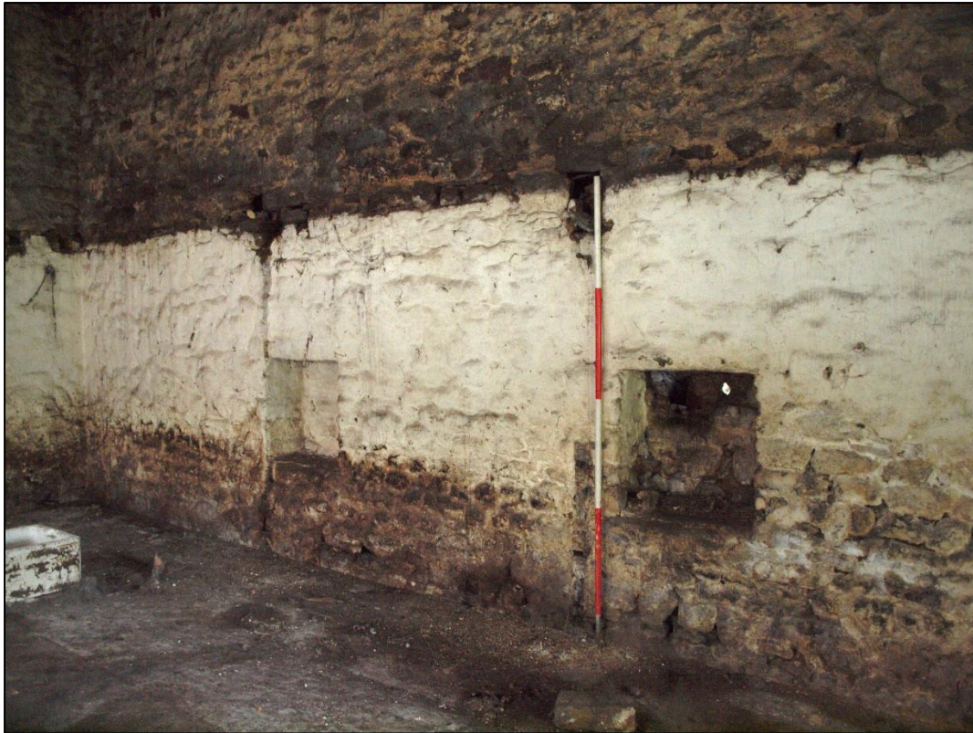
Plate 57: Blocked feeding holes in west wall
