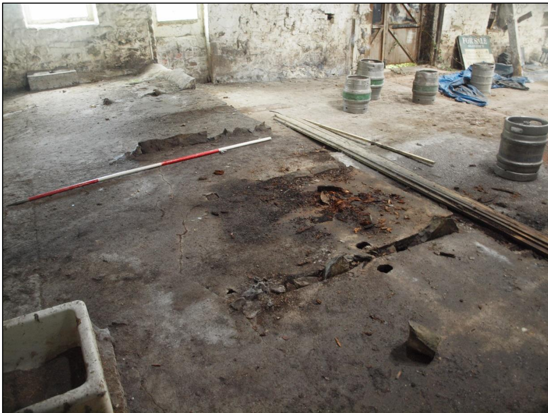
Plate 60: Scars or removed boskins in concrete floor
