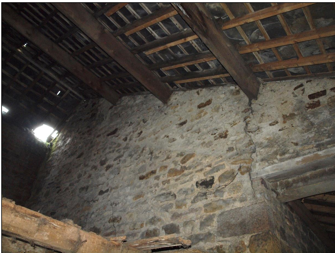
Plate 74: First floor gable showing rough joint
