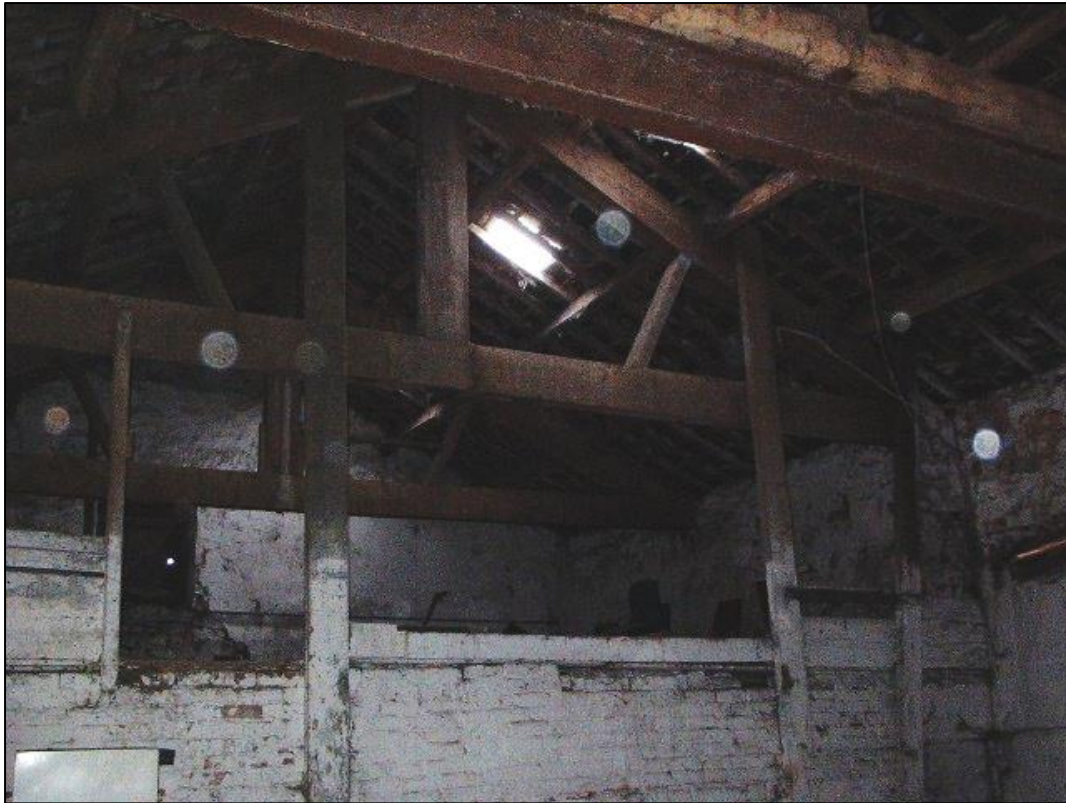
Plate 83: Interior shot c. 2011 prior to strip out (courtesy Adrian Dowd of RVBC)
