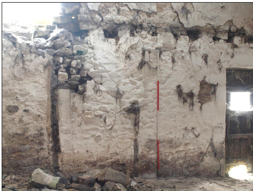
Plate 45: Scars of removed stalls in gable
