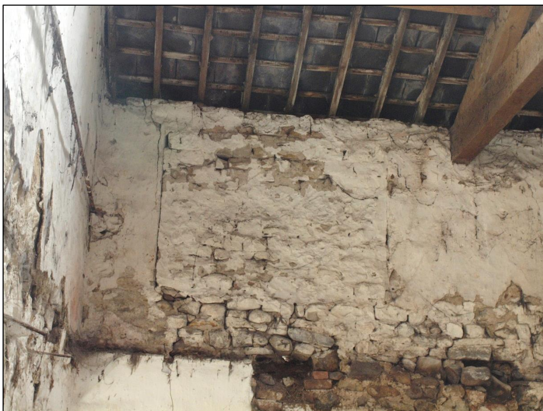
Plate 47: Blocked window shown above
