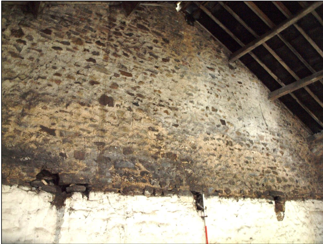
Plate 59: Detail of removed first floor joist holes an first floor of gable
