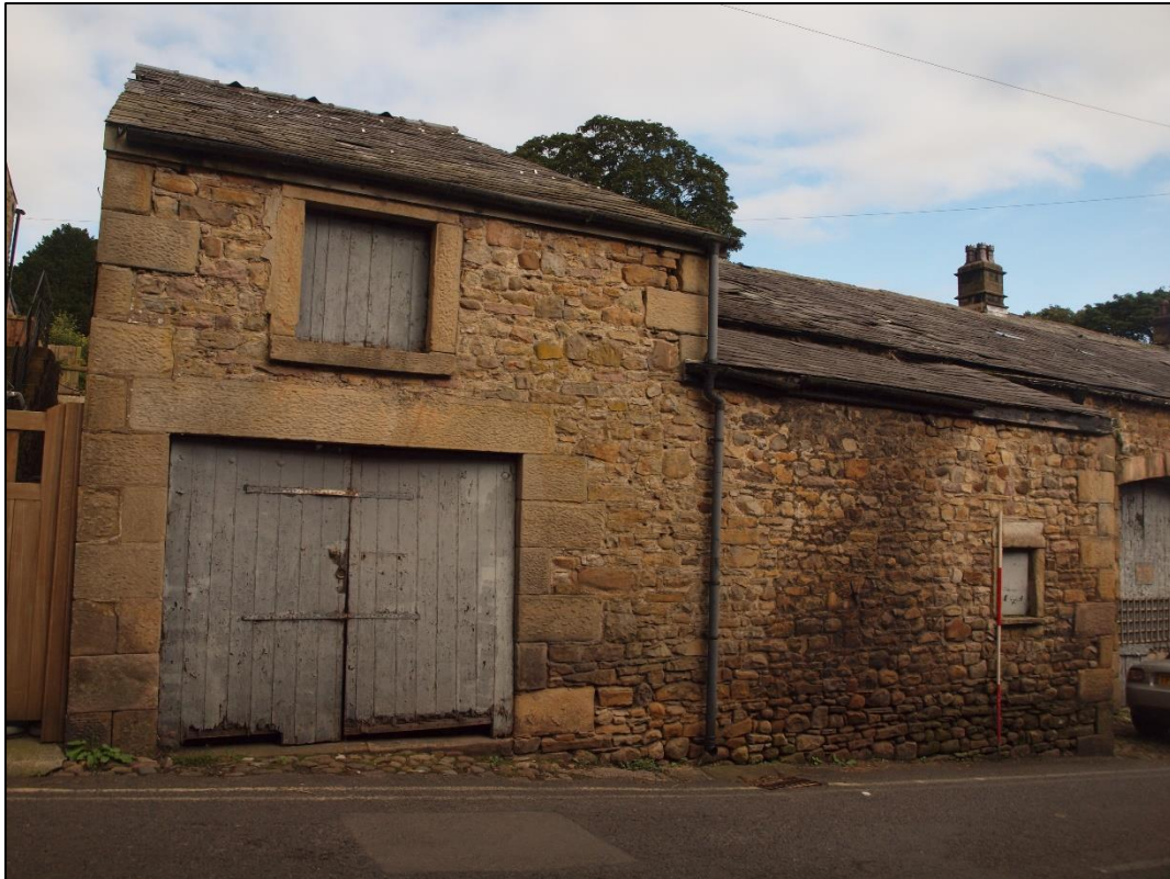
Plate 3: West end of south elevation showing out shut
