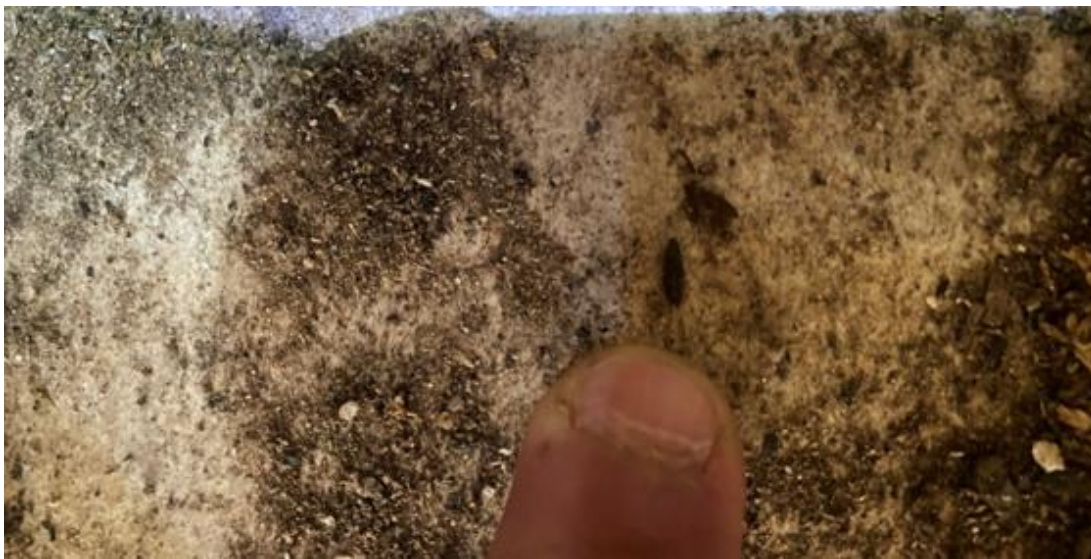
Plate 15: Evidence of bat droppings found on flat surfaces and floors (05/08/2022).
