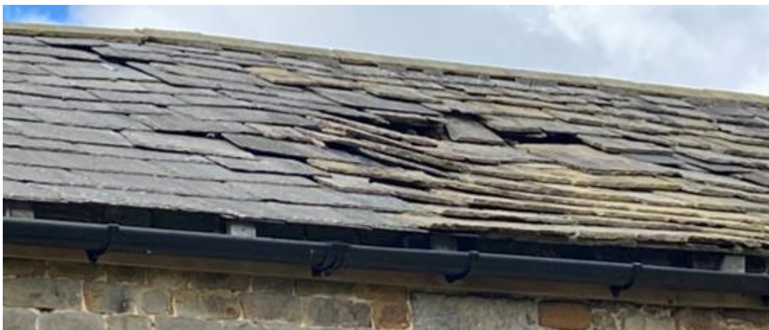
Plate 3: Large gaps under pitch tiles offered suitable roosting opportunities (05/08/2022).
