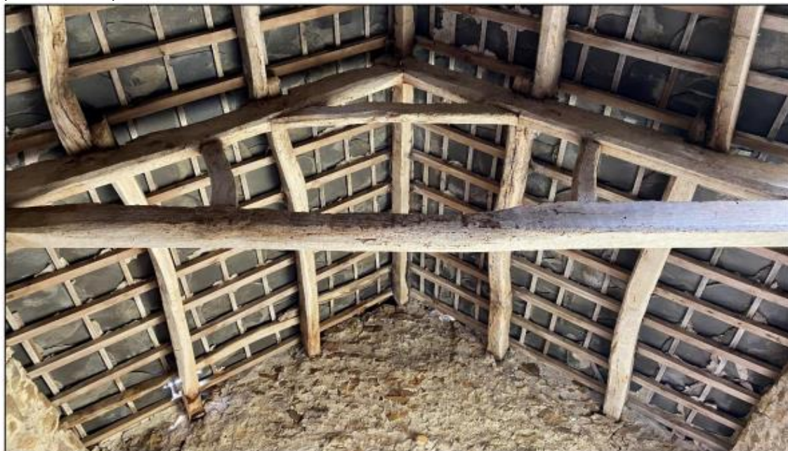
Plate 10: Timber support structures and the underside of the roof were exposed. No bats were observed (05/08/2022).
