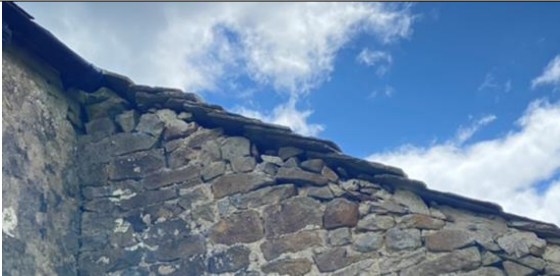
Plate 5: Gaps were apparent along the verges beneath the tiles and in the stonework, offering PRFs (05/08/2022).
