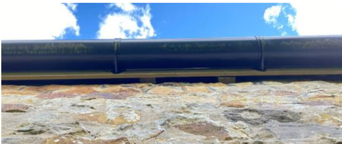
Plate 7: Gaps were visible behind fascia boards between the fascia board and the wall, offering PRFs (05/08/2022).
