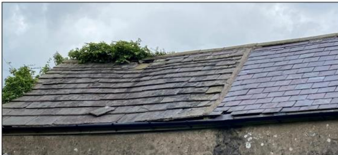
Plate 4: Slipped tiles and gaps offered PRFs (05/08/2022).
