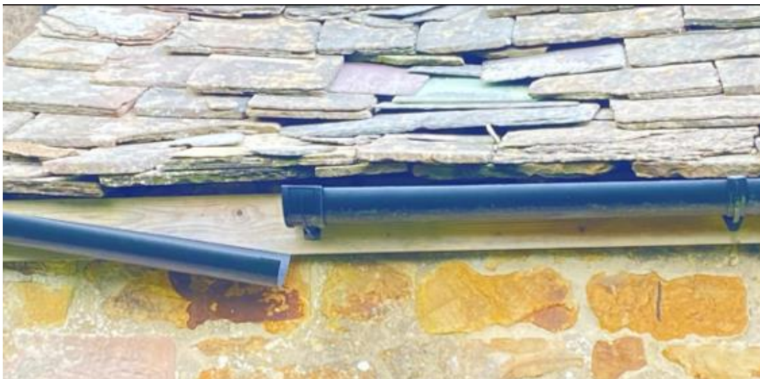
Plate 6: Gaps were apparent above the fascia boards which offered PRFs (05/08/2022).
