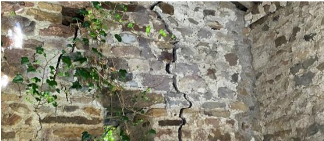
Plate 12: Internally, the walls had large cracks and gaps, offering roosting potential (05/08/2022).
