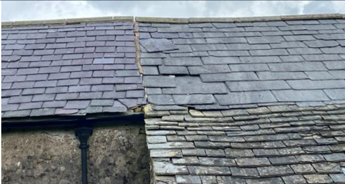
Plate 2: Pitched roof and ridges had numerous gaps and slipped tiles which offered PRFs (05/08/2022).
