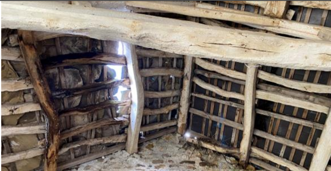
Plate 11: The roof and timber structures were in need of repair (05/08/2022).
