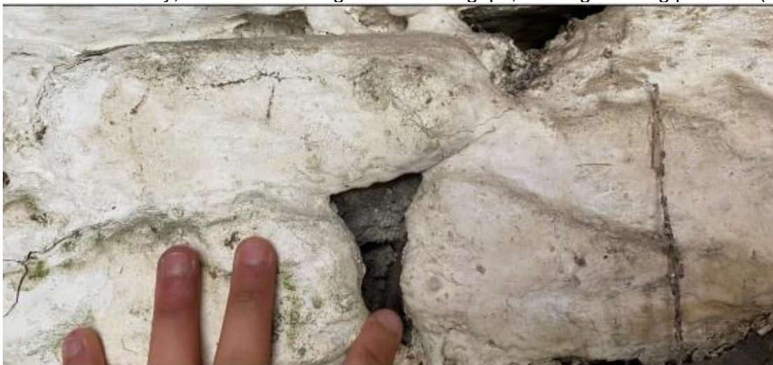
Plate 13: Large holes in the walls offered PRFs (05/08/2022).
