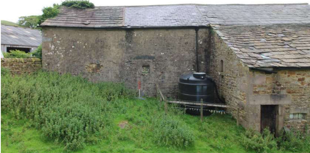
Plate 23: Western elevation of barn clad in a concrete render showing alterations to the roof slates. 1m scale
