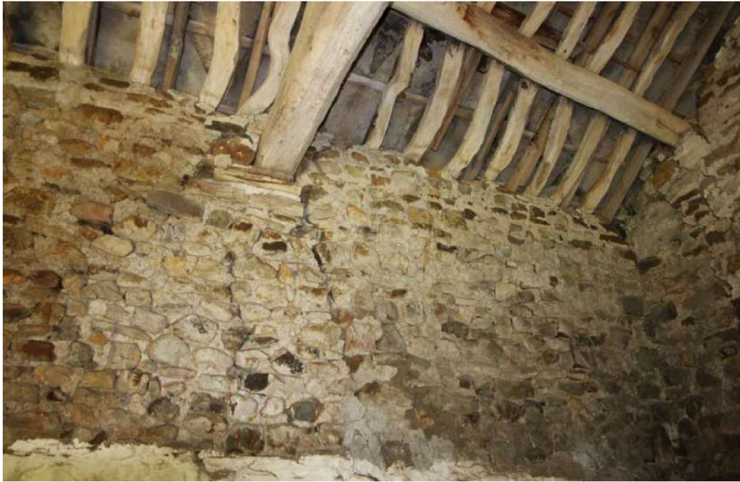
Plate 39: Vertical crack on the western wall beneath the northern queen truss (northern cell)
