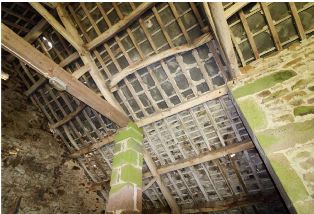
Plate 59: Gable roof (upper) and cat slide roof (lower) on western side (southern cell)
