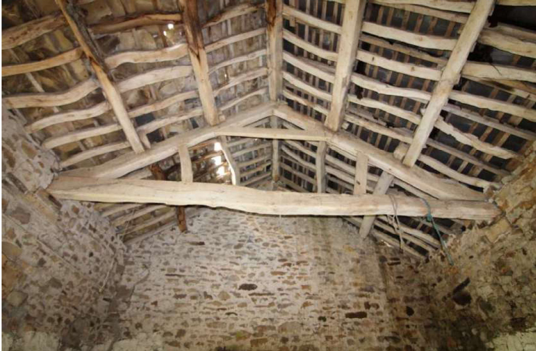
Plate 43: Queen truss at the southern end of the northern cell (one of three in the northern cell)
