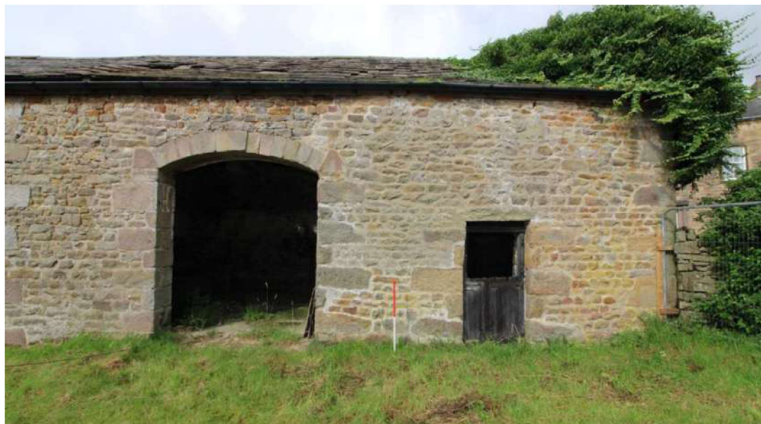
Plate 2: Northern end (cell) of principal elevation containing pedestrian width door and double-width doorway facing west. 1m scale
