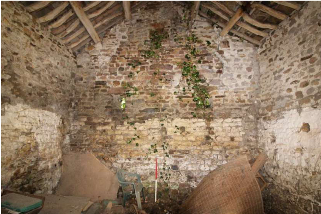
Plate 40: Northern gable end wall with vertical crack (right) (northern cell). Note the possible former roof line of an earlier building fossilised within the present gable as diagonal scars. 1m scale
