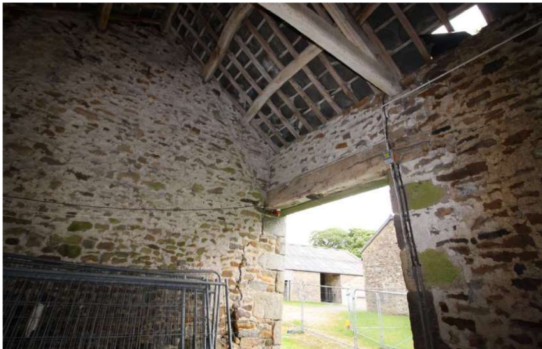
Plate 57: Vertical crack on cross-wall, facing north, (southern cell)
