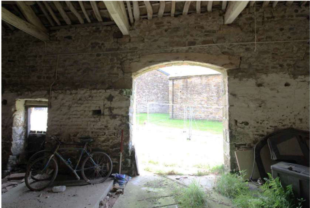
Plate 29: Interior of northern cell, facing east with double-width door, pedestrian-width door (left) and whitewashed mid-height walls. 1m scale
