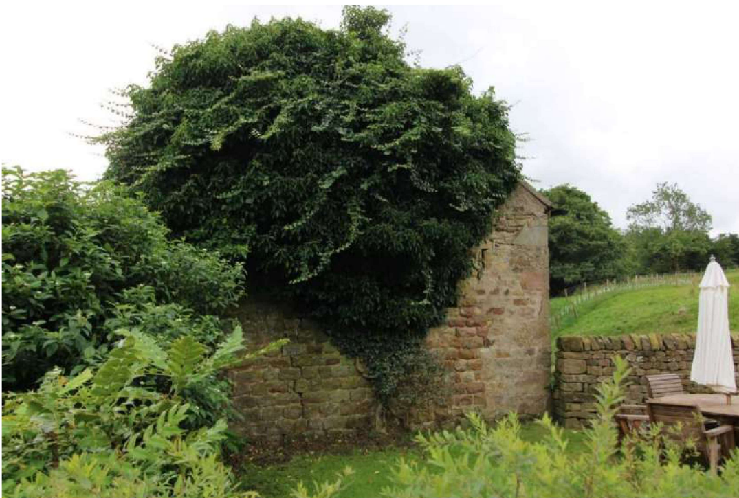
Plate 26: Northern elevation obscured by vegetation with vertical wall crack (bottom left), ventilation loop (upper right) and grey render (right)
