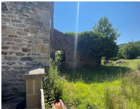
Remains of lean-to on South elevation of barn.
