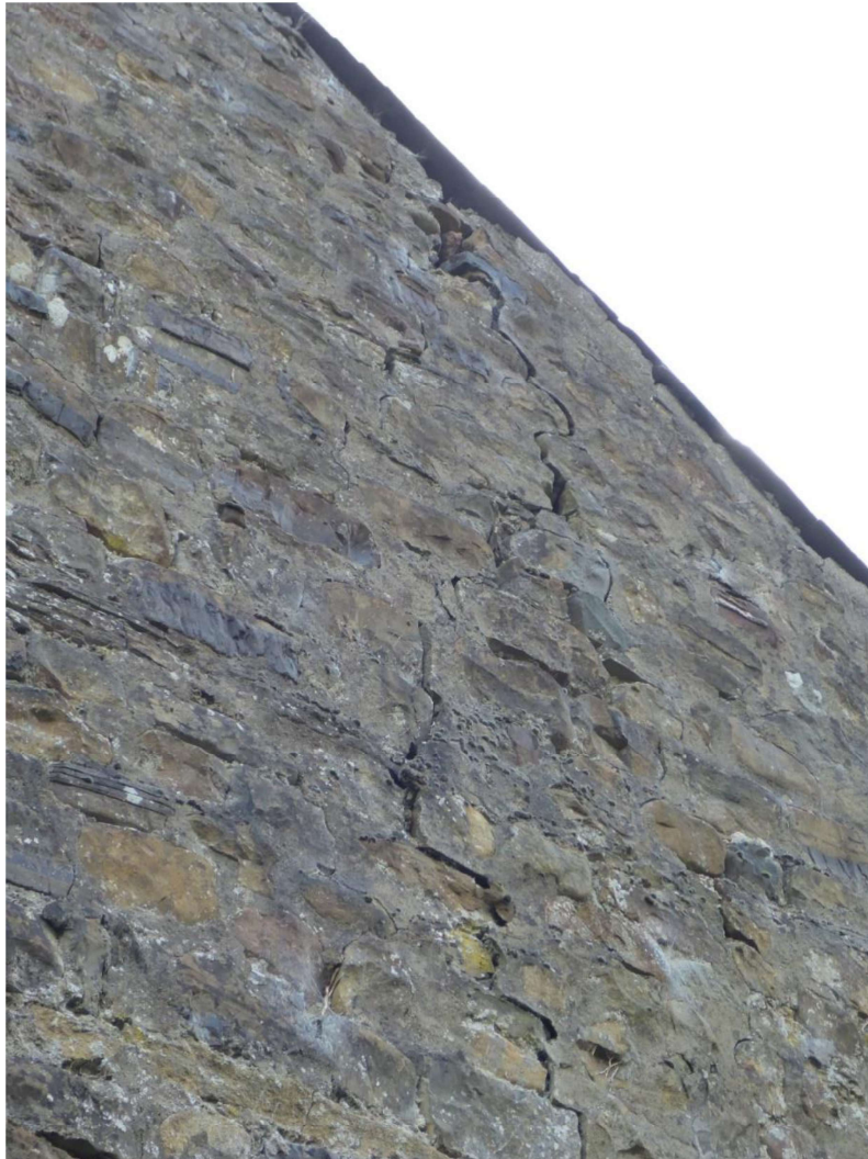
Photo 16 – Cracking on western elevation
