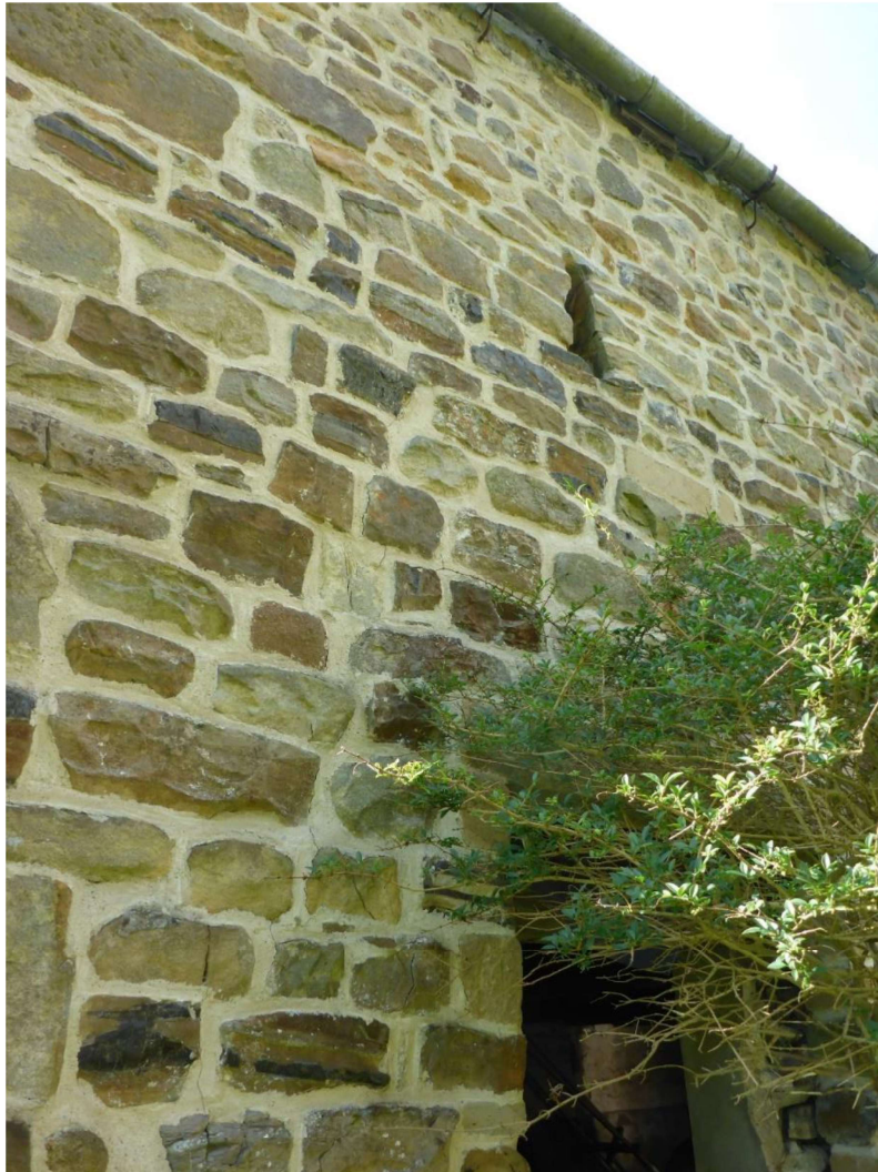
Photo 3 – Bulging masonry above front elevation window
