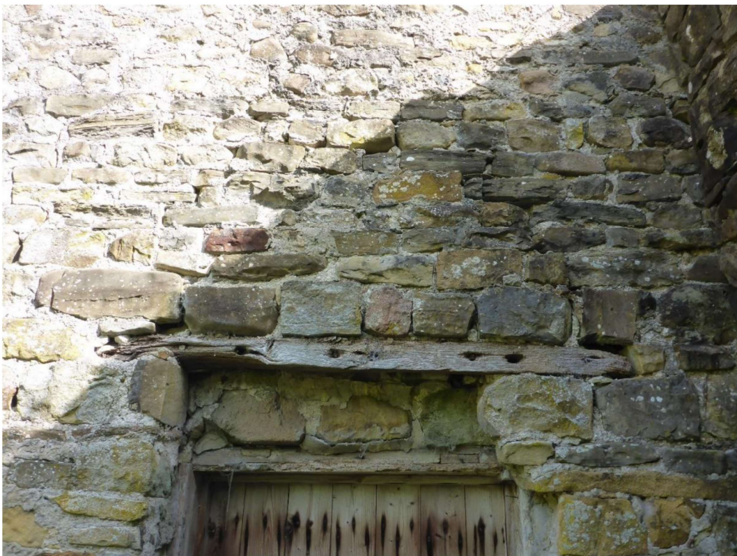
Photo 22 – Diagonal cracking over rotten timber lintel
