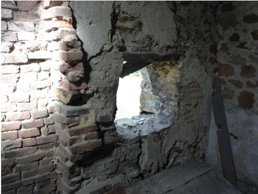
Photo 42 – Failed timber lintel at first floor level
