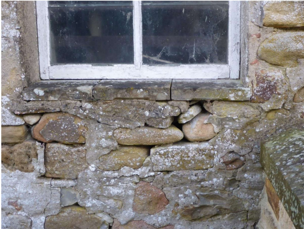
Photo 13 – missing mortar on western elevation
