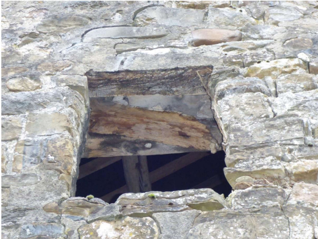
Photo 17 – Rotten timber lintel at first floor level
