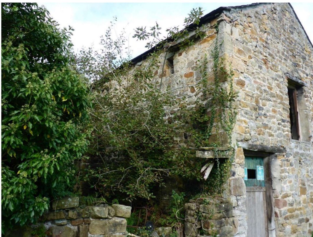
Photo 20 – Rear elevation of barn and derelict lean to
