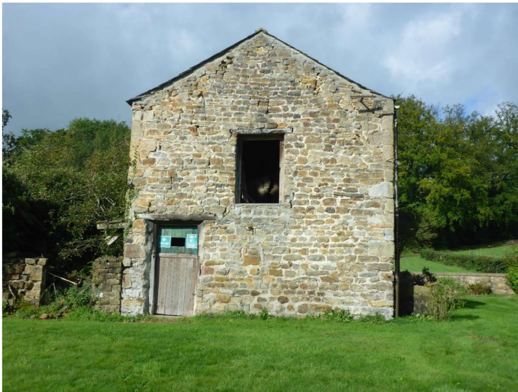
Photo 6 – Eastern elevation with missing mortar and partial repointing
