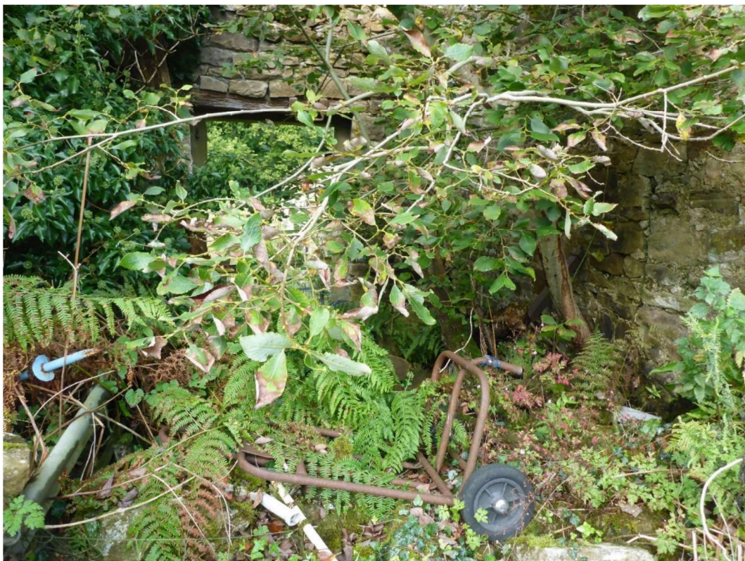
Photo 24 – Tree growing in close proximity to rear wall of barn
