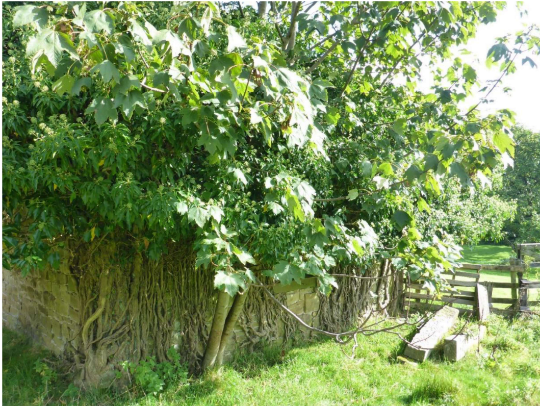
Photo 23 – Derelict lean-to to rear of barn
