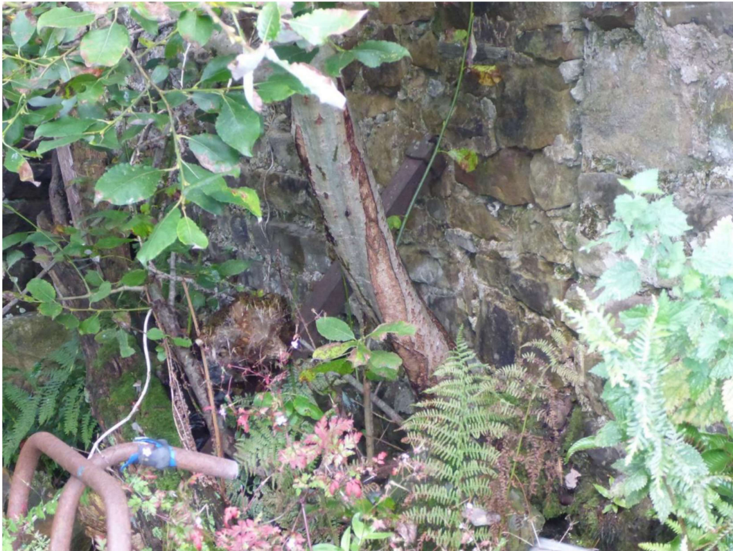
Photo 21 – Missing mortar on rear elevation
