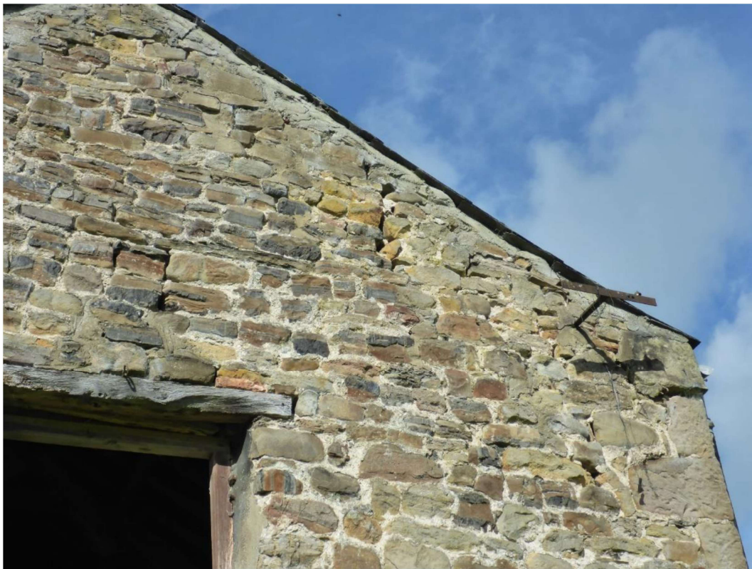
Photo 8 – Cracking and missing mortar at eaves level of eastern elevation
