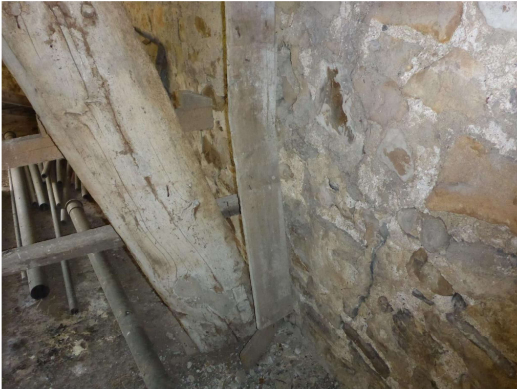
Photo 33 – Upper cruck with signs of rot and woodworm
