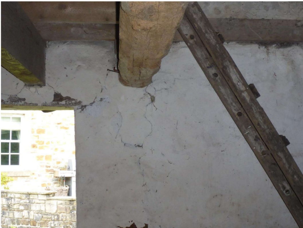
Photo 30 – Cracking beneath bearing of timber beams
