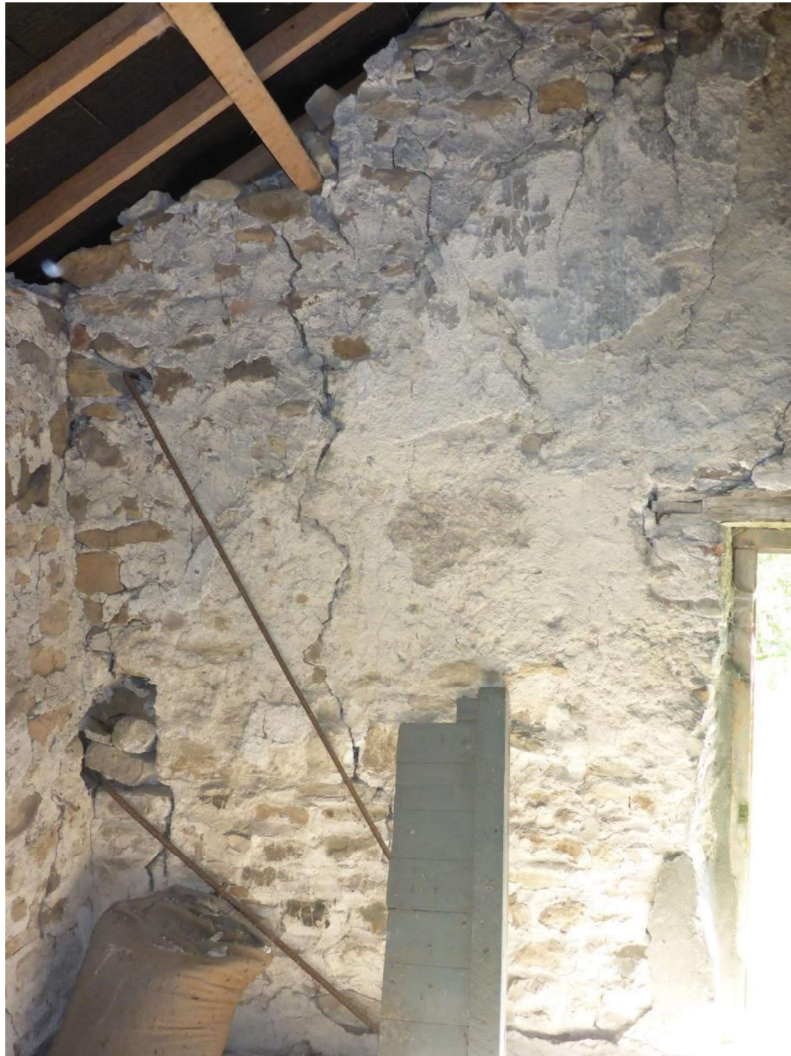
Photo 39 – Cracking in external wall at first floor level
