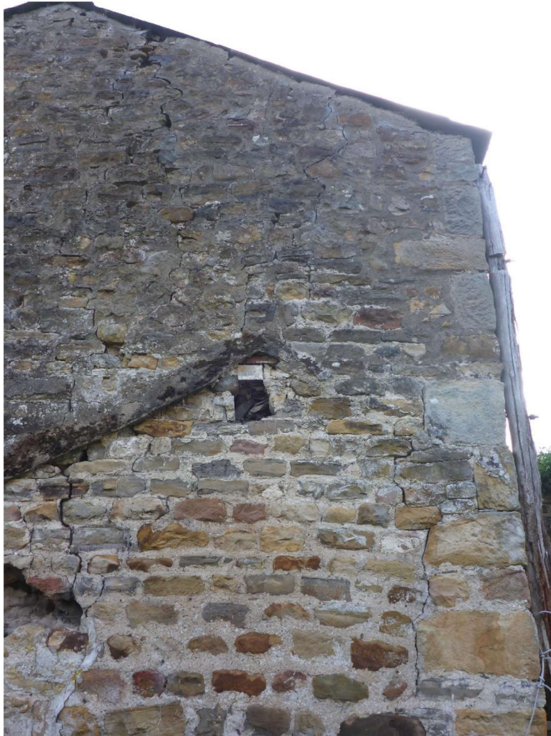
Photo 14 – Cracking on western elevation
