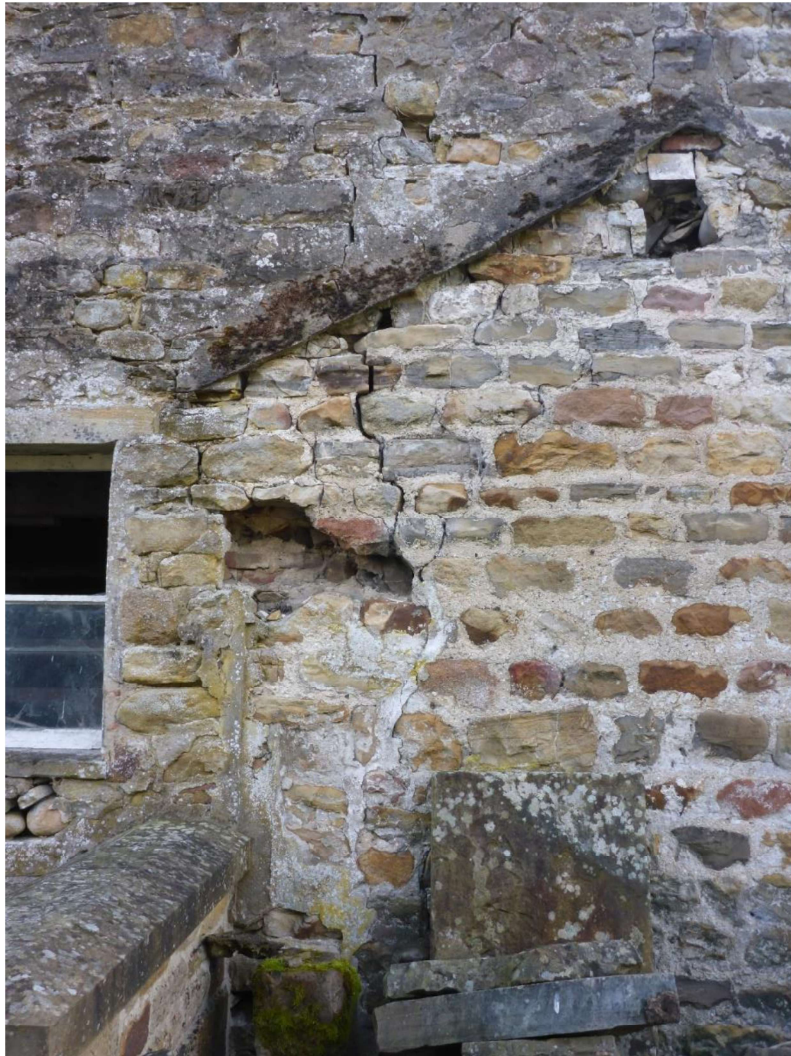
Photo 12 – Cracking and missing masonry on western elevation
