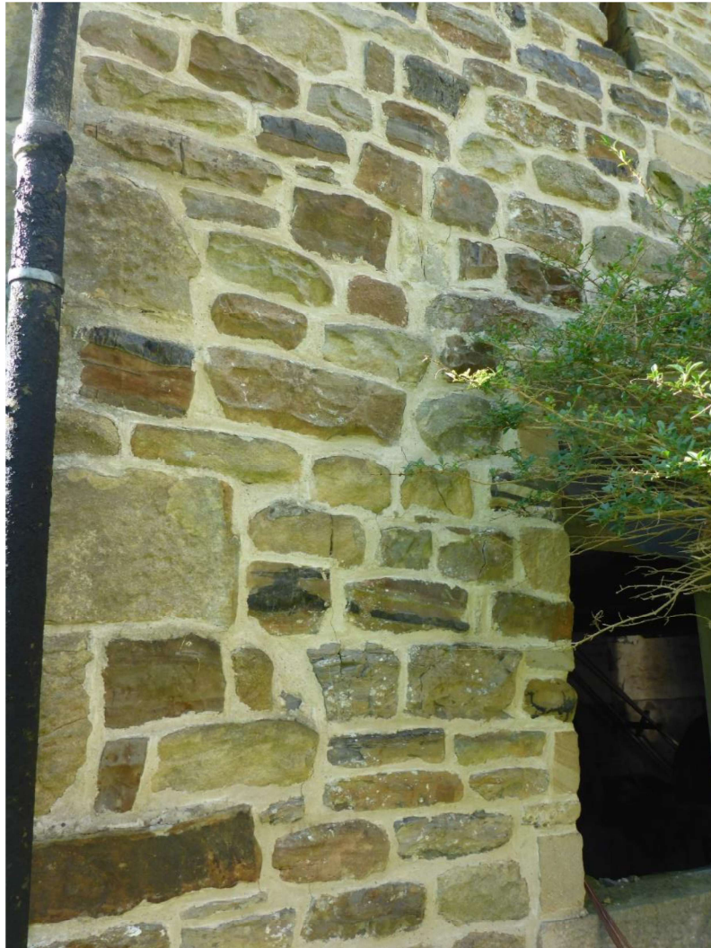
Photo 2 – Cracking around window on front elevation
