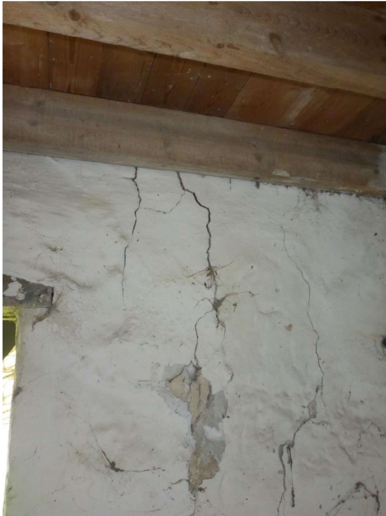
Photo 28 – Cracking in internal masonry
