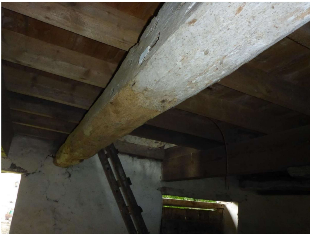
Photo 32 – Dry rot and woodworm on ceiling tie of upper cruck
