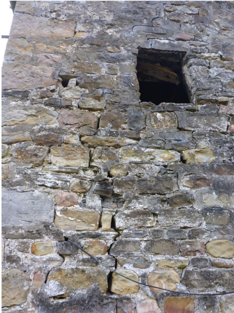
Photo 15 – Cracking on western elevation
