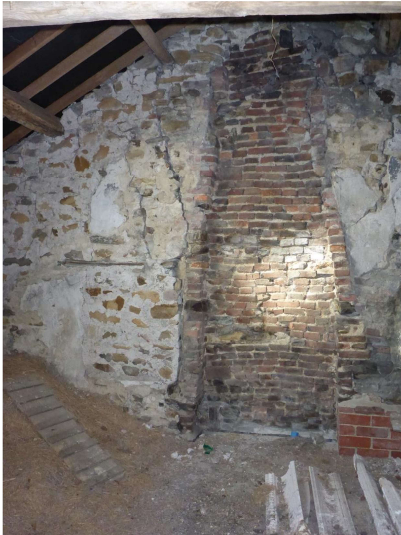
Photo 41 – Cracking in external wall at first floor level
