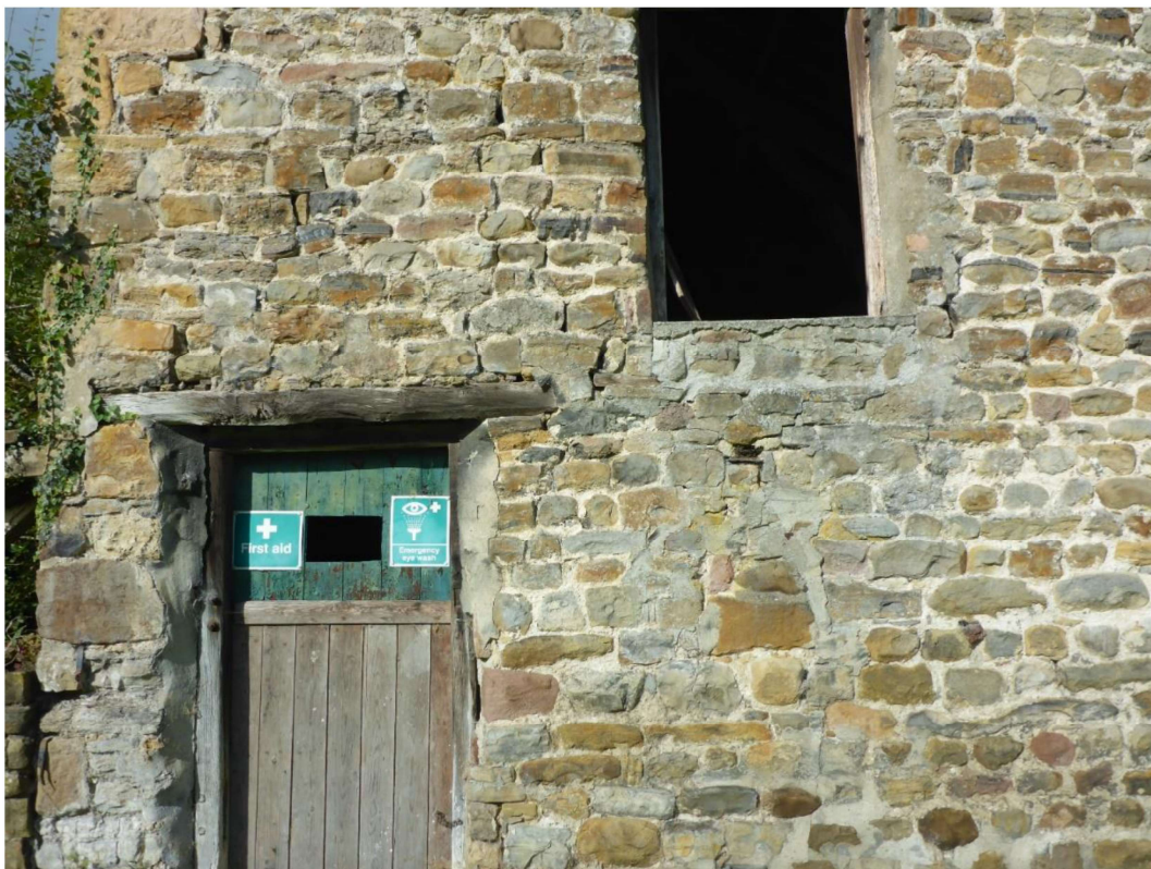
Photo 7 – Cracking around openings on eastern elevation
