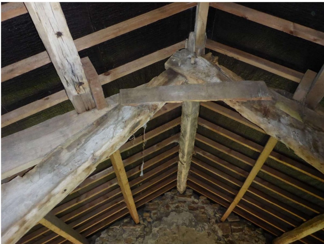
Photo 34 – Upper cruck with signs of rot and woodworm
