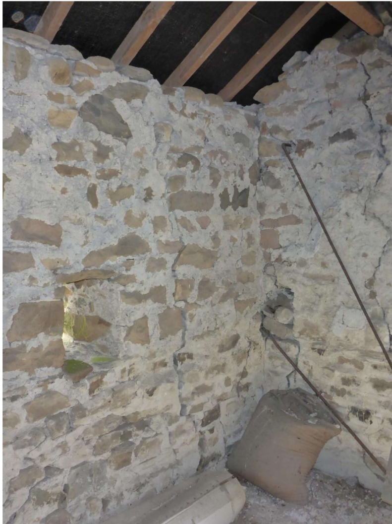
Photo 40 – Cracking in external wall at first floor level
