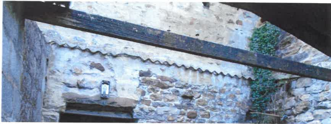
Photograph– Showing the condition of the roof structure to the Lean to.
