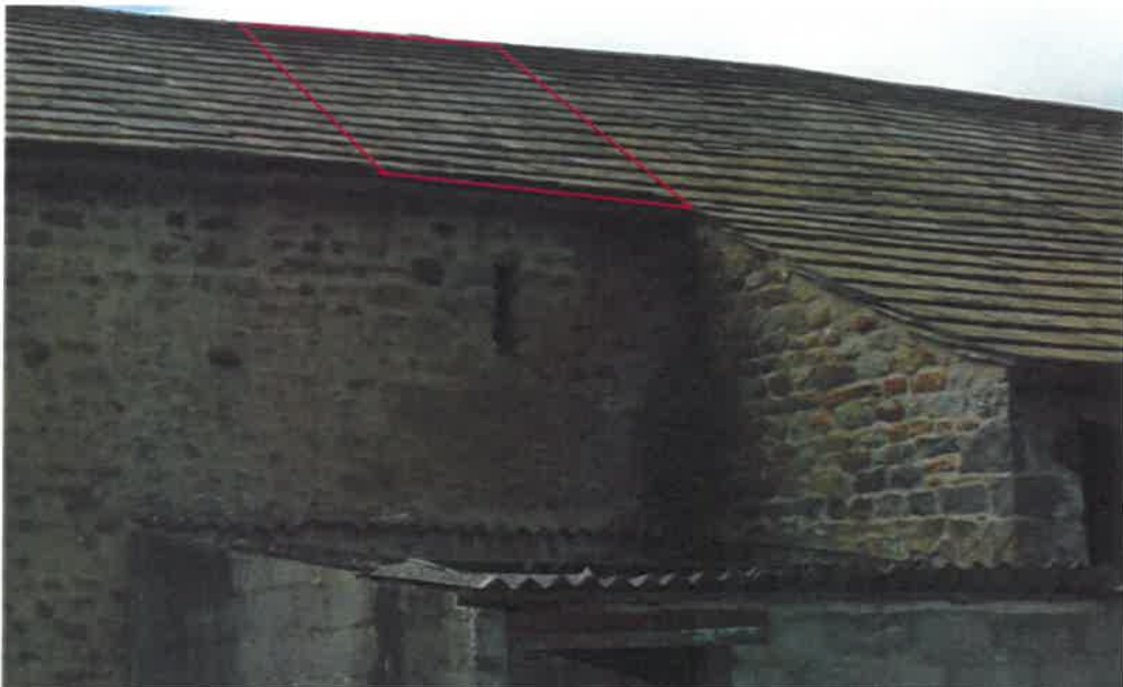
Photograph– Showing the condition of the roof to the main barn ( North west elevation) .( section being affected by the conversion highlighted in red)
