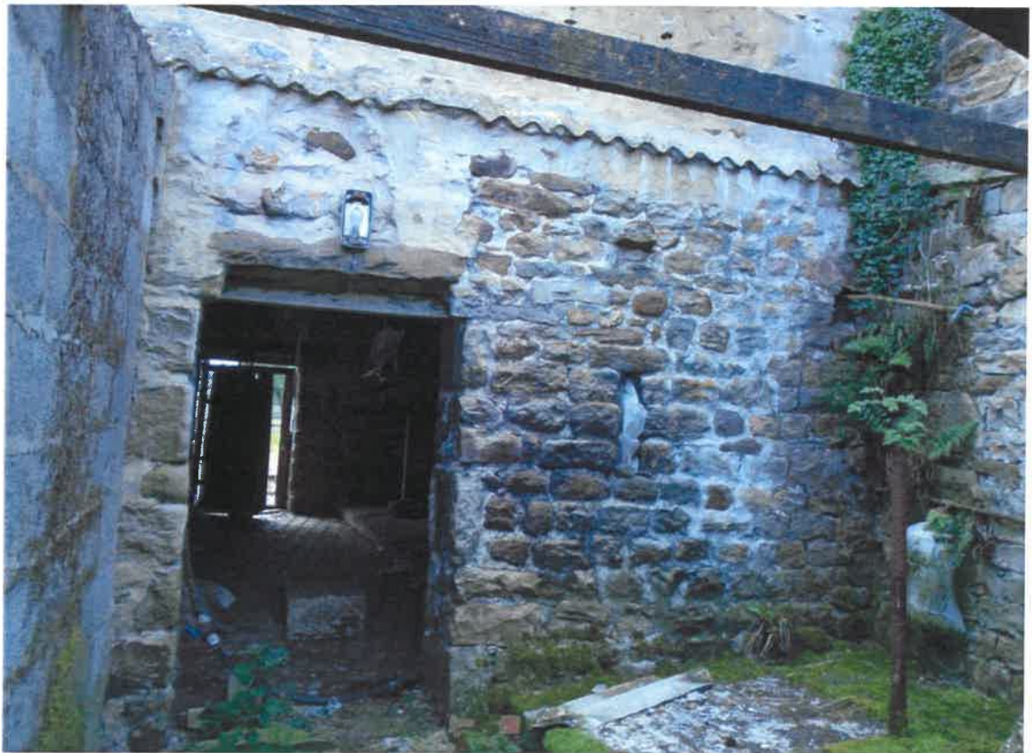
Photograph – Illustrating the condition rear wall within the lean to.
