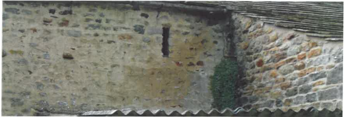
Photograph– Illustrating the condition Rear wall above the Lean to.
