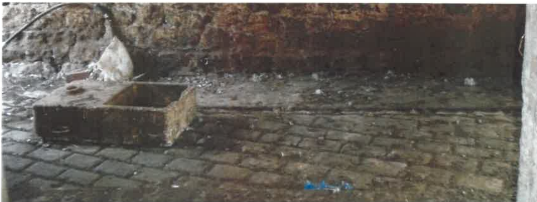
Photograph– Illustrating the condition of the internal floor .
