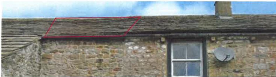
Photograph– Showing the condition of the roof to the main barn ( south east elevation) .( section being affected by the conversion highlighted in red)
