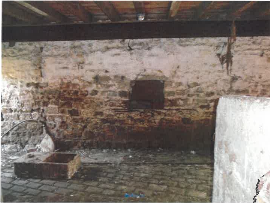
Photograph– Illustrating the condition of the internal wall adjacent to the house.
