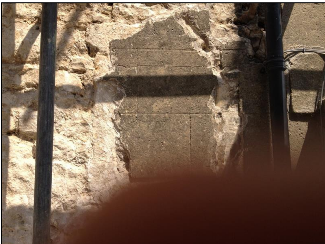
PLI 5: Photograph showing the former window to the ground floor of the west gable elevation, at the south end of the elevation.
