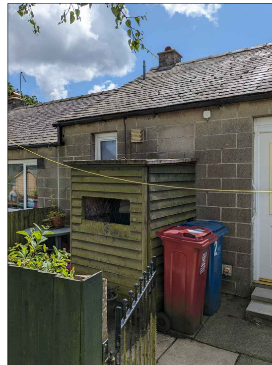
Photos of ASHP as Existing
