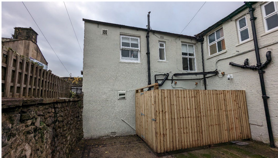
Figure 10 - Rear elevation which has been pebble-dashed and a number of openings infilled.
