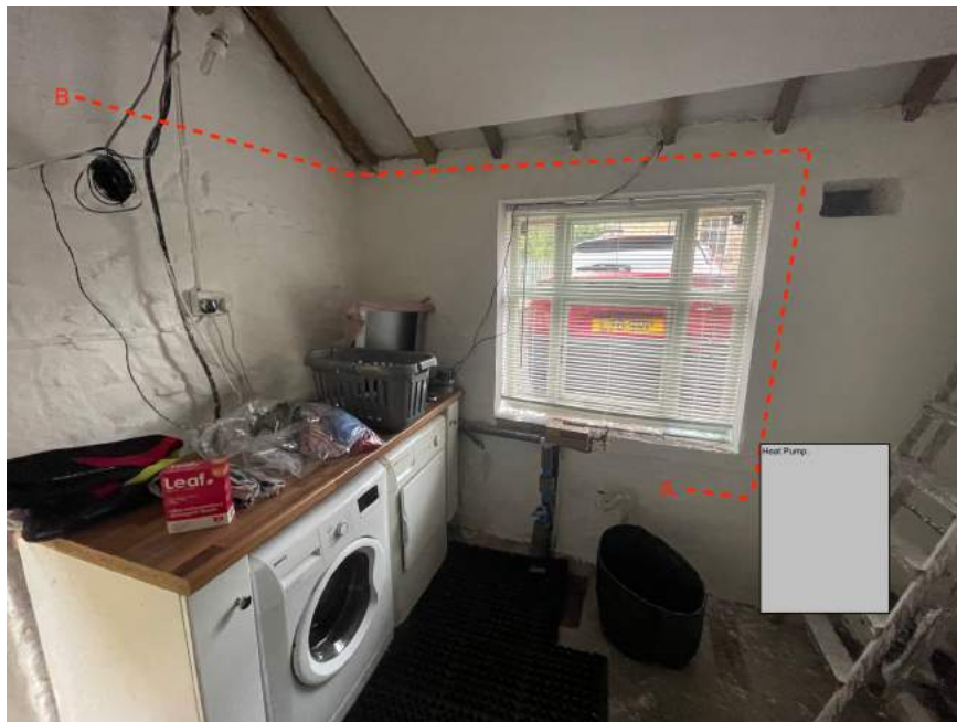
The inside of the wash-house where the heat pump will be located.
