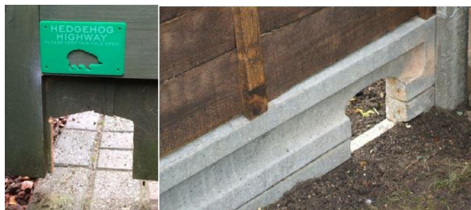
Insert 4: Showing wildlife access gap within fencing
