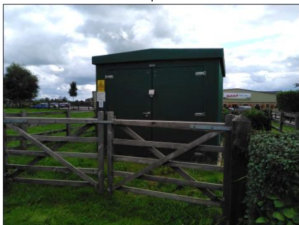
Photo 5: Electricity sub-station (Building 1)
