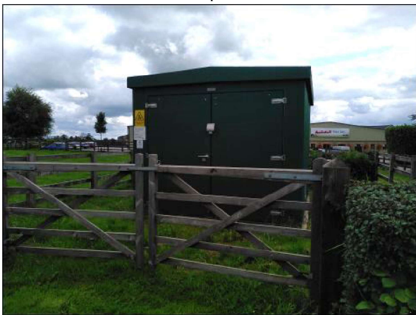
Photo 5: Electricity sub-station (Building 1)
