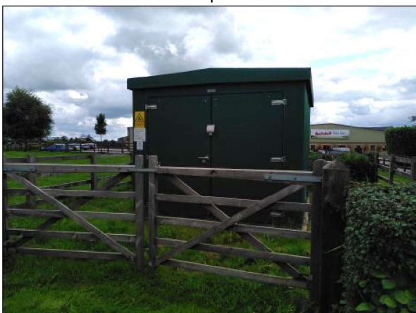
Photo 5: Electricity sub-station (Building 1)
