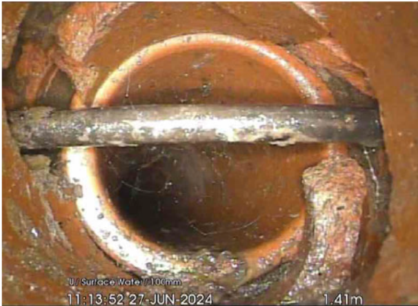
FWG1X_13068a09-f90e-40b2-9885-353f1bf6be3d_20240701_112917_688.jpg, 00:00:32, 1.41 m Other obstacles, external pipe or cable from 12 o'clock to 12
