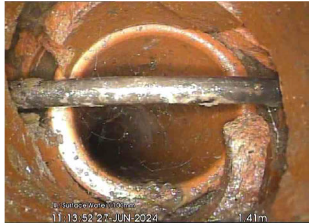
FWG1X_6a409a7f-89e2-47d4-abb2-d818c7c07e1d_20240701_112946_865.jpg, 00:00:32, 1.41 m Survey abandoned, Unable to pass intruding pipe
