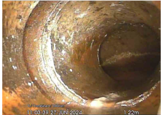
FW1X_ec44b91d-e102-47e8-9e84-b4a8b3c1812b_20240701_112000_699.jpg, 00:00:16, 1.22 m Joint displaced, large
