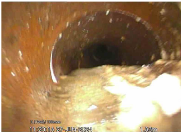
FWMH2X_0a091bb0-7b5e-44bd-9973-3e0f53a431e1_20240701_114023_809.jpg, 00:00:07, 1.33 m Settled deposits, hard or compacted, 50% cross-sectional area
