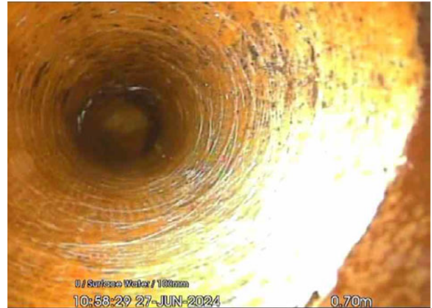
SVP2X_871d0ace-c1fc-41ca-9613-4776404a0f56_20240701_111412_873.jpg, 00:00:21, 0.70 m Point repair, localised lining from 12 o'clock to 12 o'clock
