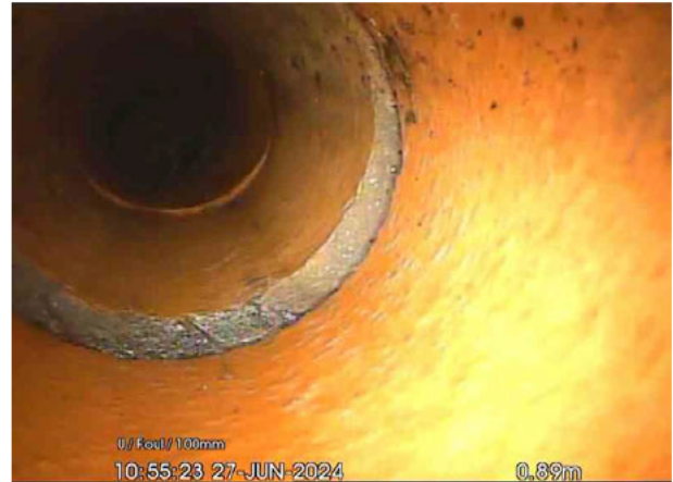
SVP1X_c90036b4-9e08-4e23-b7a7-73cc8126e8dd_20240701_112531_593.jpg, 00:00:09, 0.89 m Joint displaced, large
