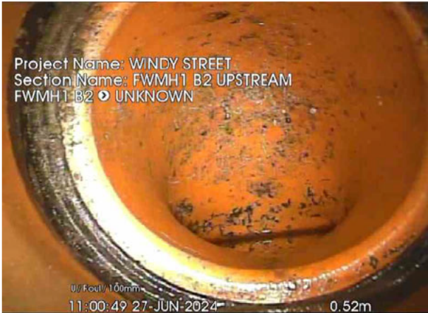
FWGX_a51170b8-ac1c-4053-b36b-cf994d9bccd2_20240701_111649_209.jpg, 00:00:04, 0.52 m Open joint, large
