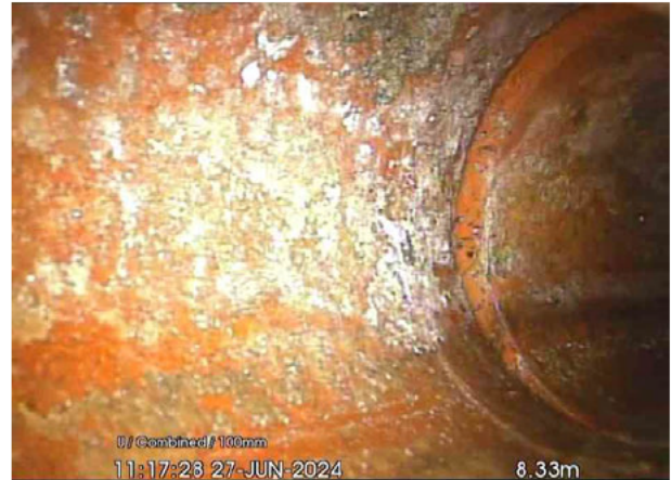
FWMH2 X_58f063ce-d040-4570-b500-051683946195_20240701_113626_403.jpg, 00:01:06, 8.33 m
