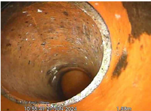
SVP1X_7b0a12f3-0cab-4732-908d-03a4a77b8cf2_20240701_112559_073.jpg, 00:00:21, 1.58 m Joint displaced, medium
