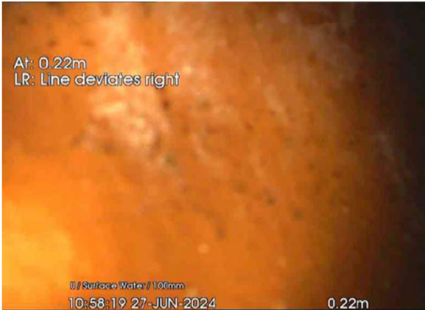
SVP2X_25230407-3007-425f-b237-ed0644a78be8_20240701_111332_401.jpg, 00:00:12, 0.20 m Line deviates right
