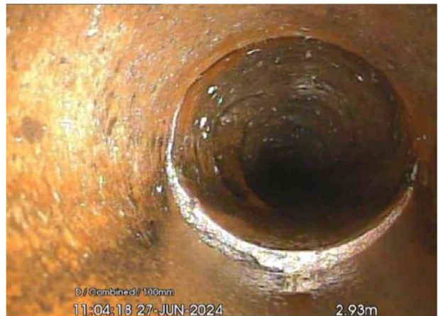
FW1X_aa08e7da-3798-4b9c-ad8d-91663a9c2861_20240701_112055_994.jpg, 00:00:38, 2.90 m Joint displaced, medium
