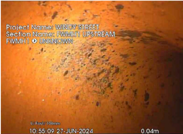
SVP1X_31c22fda-5397-4197-b733-d6dc68de90a3_20240701_112509_601.jpg, 00:00:01, 0.04 m Line deviates right
