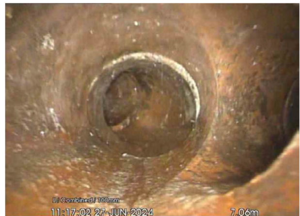
FWMH2 X_9fe8d35f-da92-4cef-97a1-d7eff22a05f4_20240701_113533 _833.jpg, 00:00:51, 7.00 m
