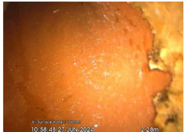
SVP2X_8708c846-7028-4578-84ff-810c593bc1db_20240701_111457_241.jpg, 00:00:35, 2.28 m Line deviates up
