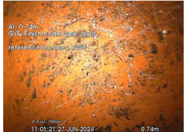
FWGX_61004805-0dcf-4ec8-819c-748c6d05e268_20240701_111809_826.jpg, 00:00:22, 0.74 m Finish node, gully, reference: RWG1
