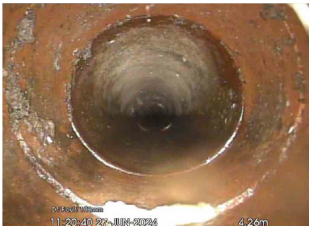
FWMH2X_59358f4b-3add-4a31-b431-0bdc0da22a33_20240701_114120_001.jpg, 00:00:31, 4.26 m Crack, circumferential at joint from 12 o'clock to 12 o'clock
