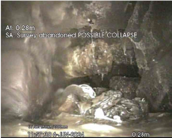
LAS MH1 UPSTREAM_0-28m_115738.jpg, 00:00:47, 0.28 m Survey abandoned, POSSIBLE COLLAPSE CULVERT
