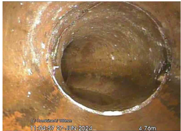
FW1X_c771fd82-17fb-45cb-a40e-eb2a5892b47d_20240701_112208_339.jpg, 00:01:02, 4.76 m Fracture, circumferential at joint from 9 o'clock to 12 o'clock
