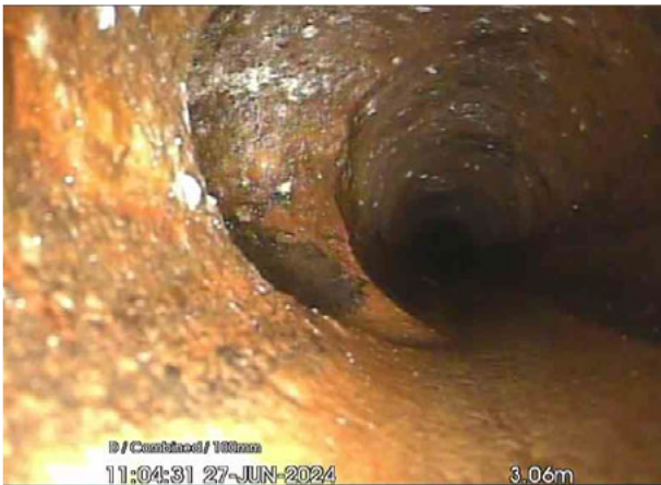
FW1X_771ea0ea-f22e-4449-8a53-de24fa63c19f_20240701_12117_304.jpg, 00:00:45, 3.00 m Junction at 9 o'clock, diameter: 100mm
