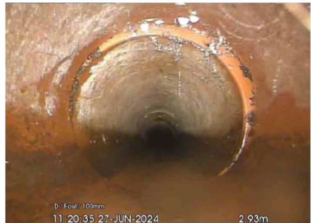
FWMH2X_fd47bc22-ee4e-4841-85af-162f50f26e8e_20240701_114056_121.jpg, 00:00:25, 2.93 m Joint displaced, medium
