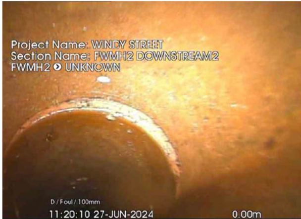
FWMH2X_7c2f1987-98f2-4a86-b2b9-3a70ec7d8762_20240701_113938_049.jpg, 00:00:01, 0.00 m Line deviates down
