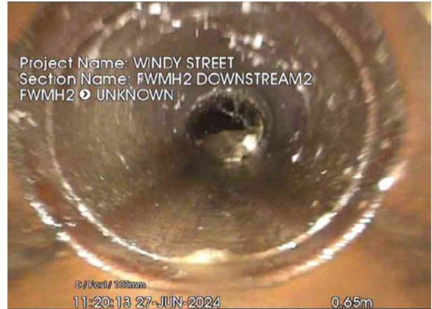
FWMH2X_ff75e588-162b-4416-8182-dc0325489872_20240701_114001_280.jpg, 00:00:04, 0.65 m Fracture, circumferential at joint from 12 o'clock to 12 o'clock
