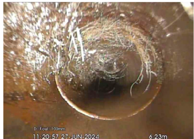
FWMH2X_4740529b-41c2-4d16-a6a0-55832721220a_20240701_114143_169.jpg, 00:00:41, 6.23 m Roots, fine at joint
