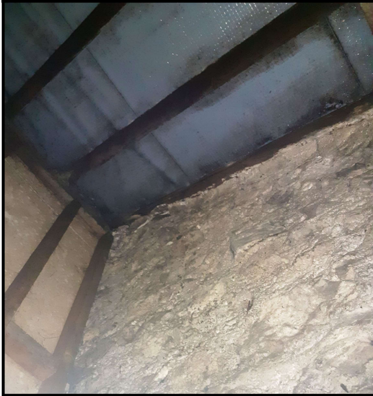
Roof void – showing timber dividing wall, stone gable wall and underside of roof
