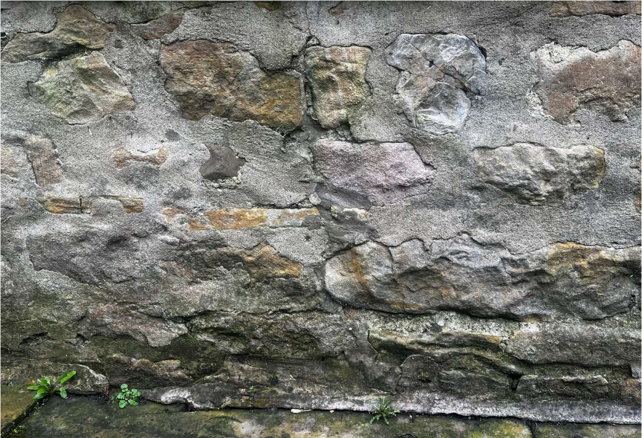
Photo 2 – Cement mortar covering large portions of the sandstone
