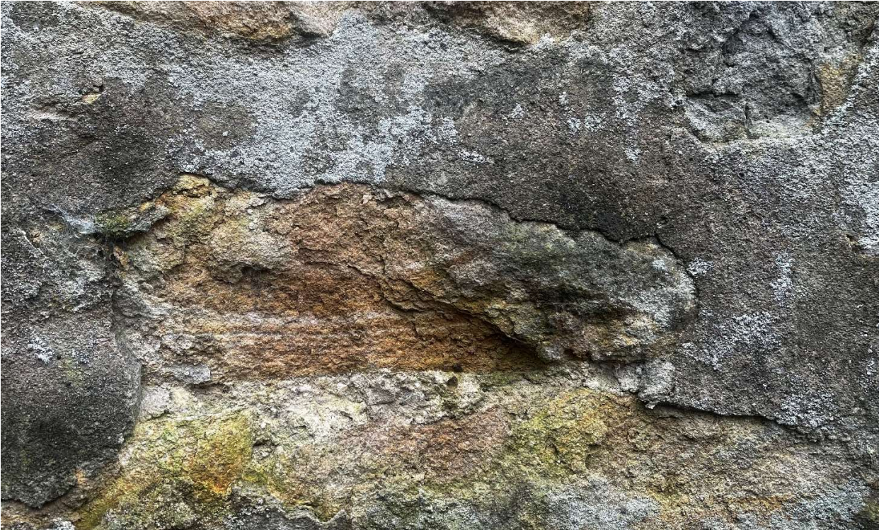
Photo 3 - Damage to sandstone due to cement based mortar covering face of stonework
