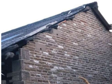
Example of Forticrete boxes in situ
