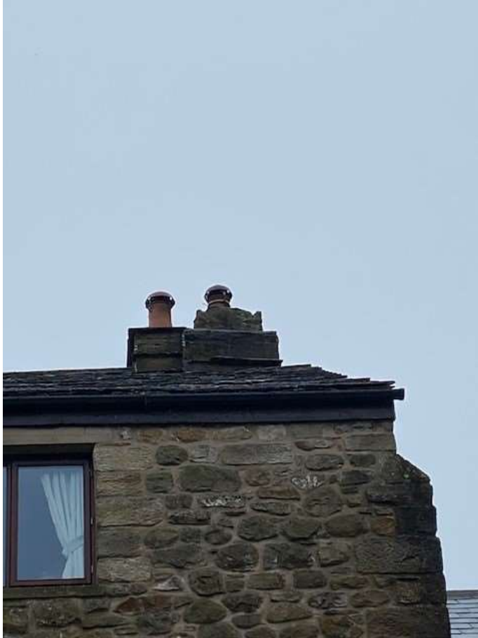
Photo of existing chimney requiring repair.
