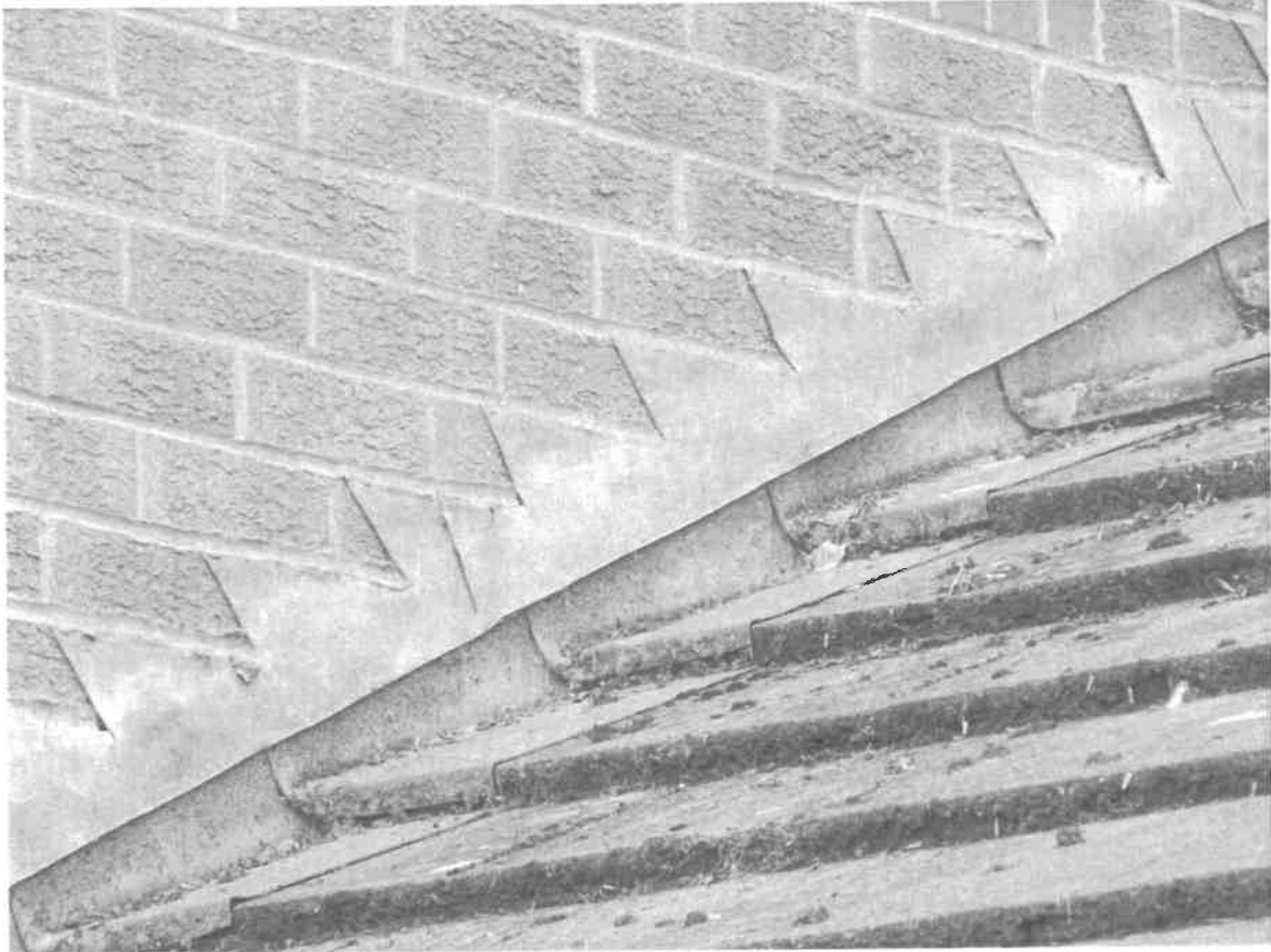
5 – Lead flashing is fitted tightly with no suitable gaps.
