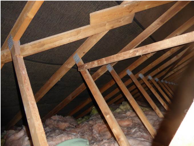
Loft space of bungalow, lined with bitumen roofing felt below concrete tiles.
