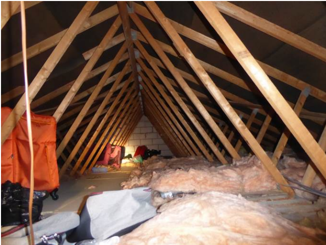
Loft space of bungalow, lined with bitumen roofing felt below concrete tiles.
