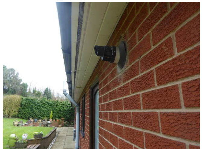
Rear western elevation of existing bungalow, soffits are tight fitting to the brickwork.
