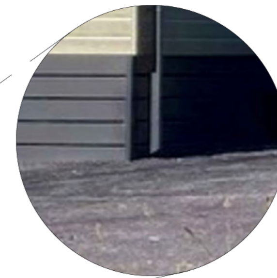
Enlarged image showing caravan rainwater pipes curtailed above ground and surface water allowed to drain directly onto permeable gravel area
