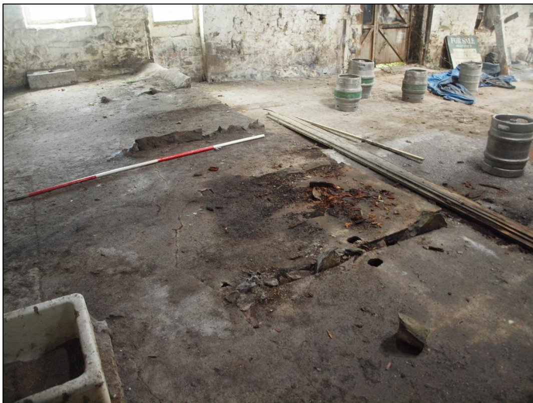
Plate 60: Scars or removed boskins in concrete floor
