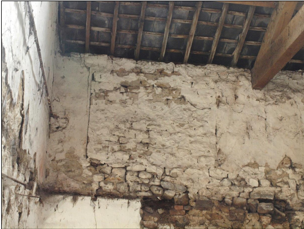
Plate 47: Blocked window shown above
