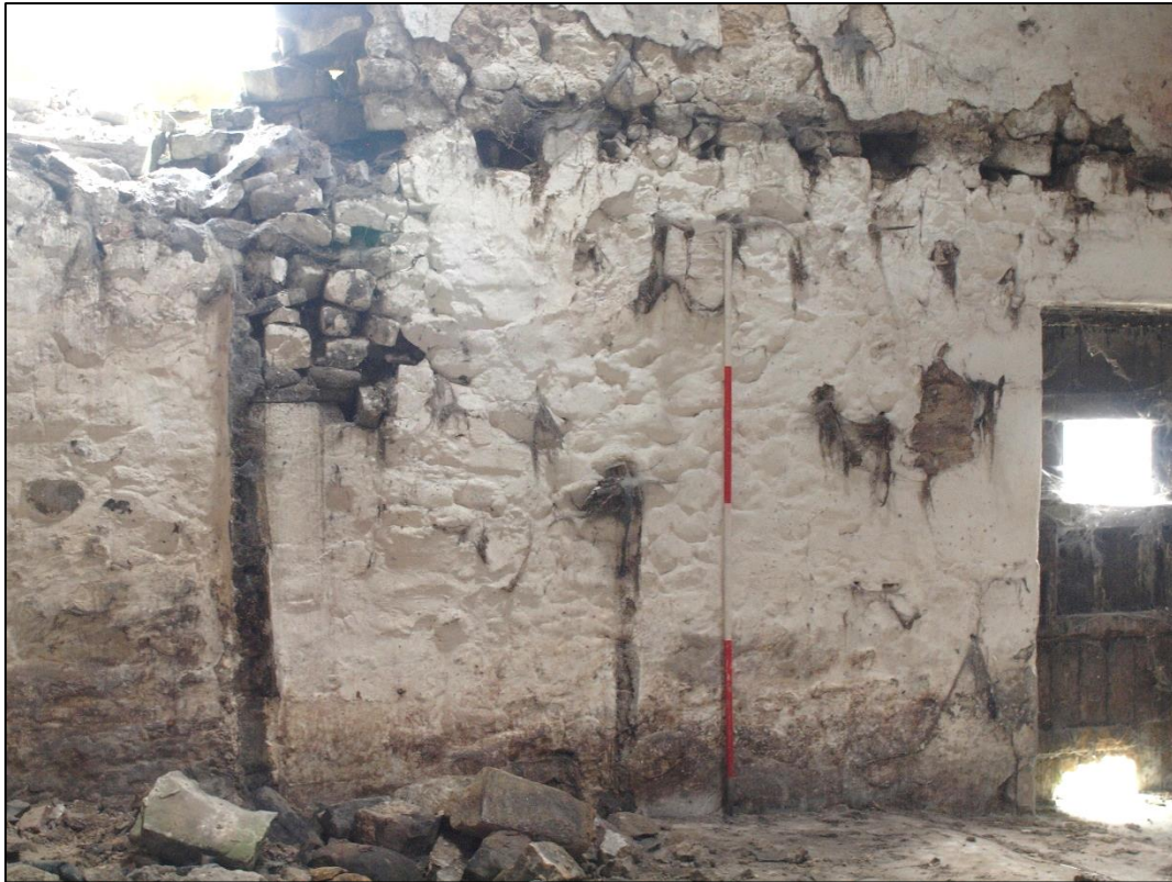
Plate 45: Scars of removed stalls in gable
