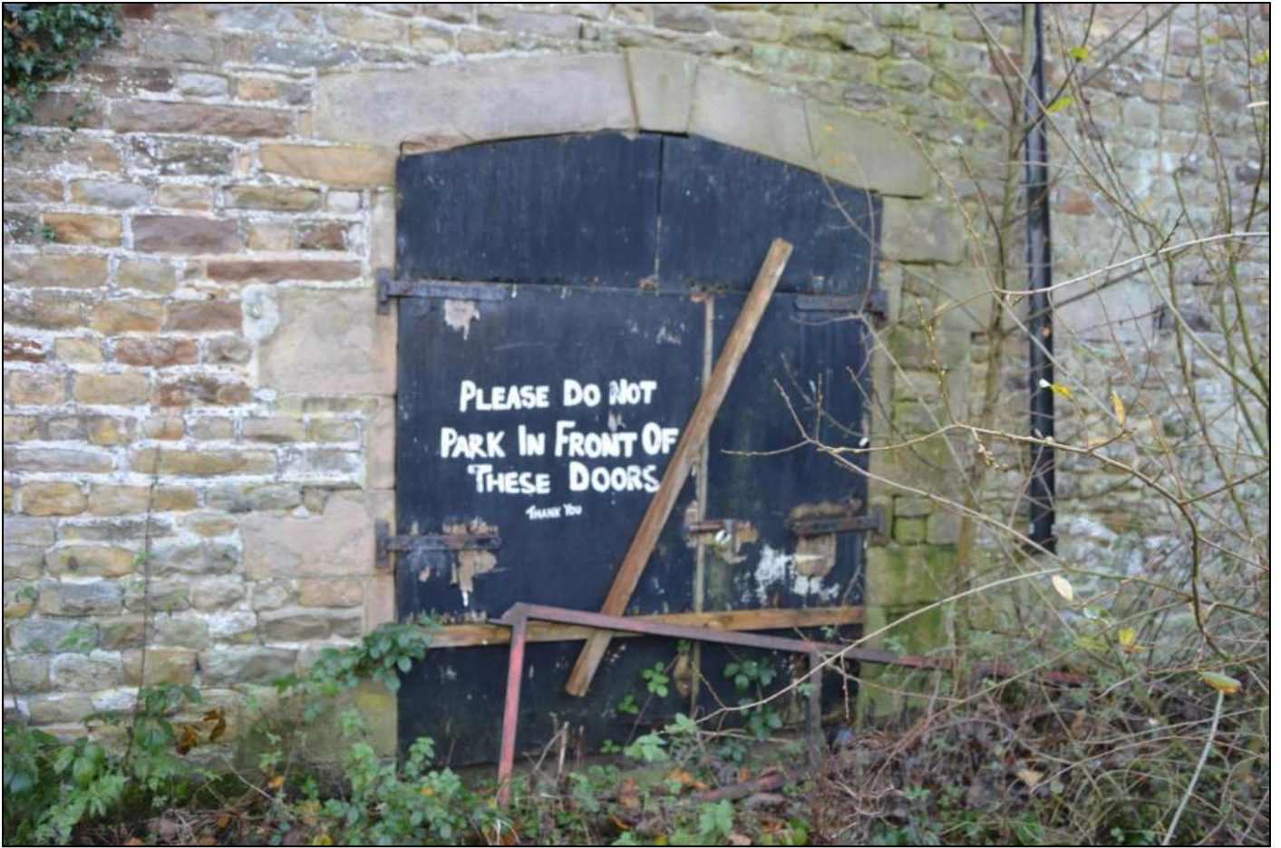
PL81: View of the former crat entry to the north west elevation of the barn.
