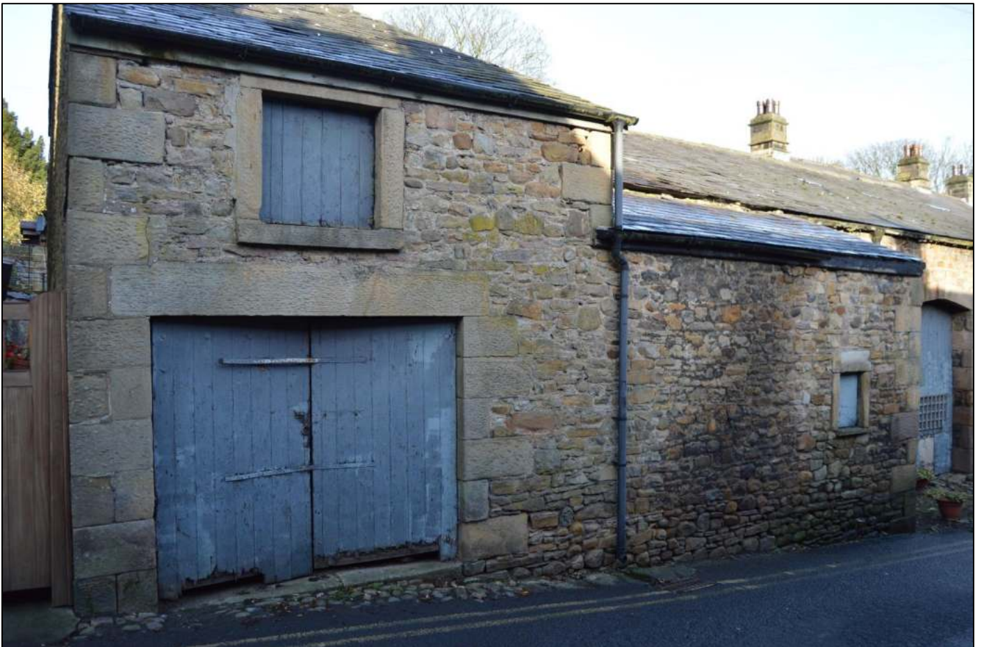
PL76: View of the south east facing elevation of the 19 th century addition to the barn.
