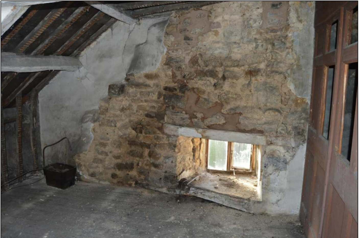
PL69: View of the chimney flues and former mullioned window to the south west wall of the attic.
