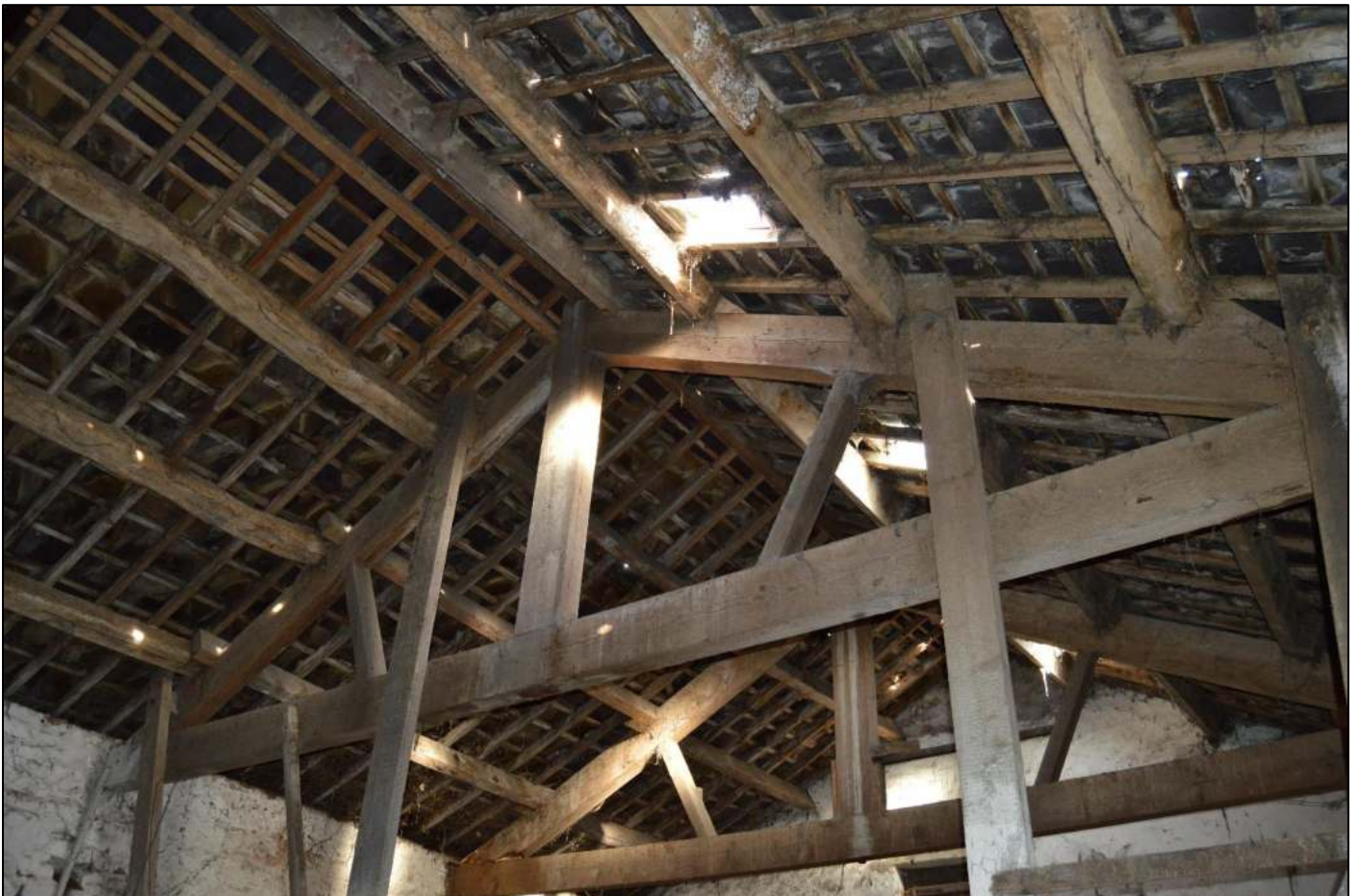
PL88: View of the 2no replacement roof trusses to the north end of the barn.
