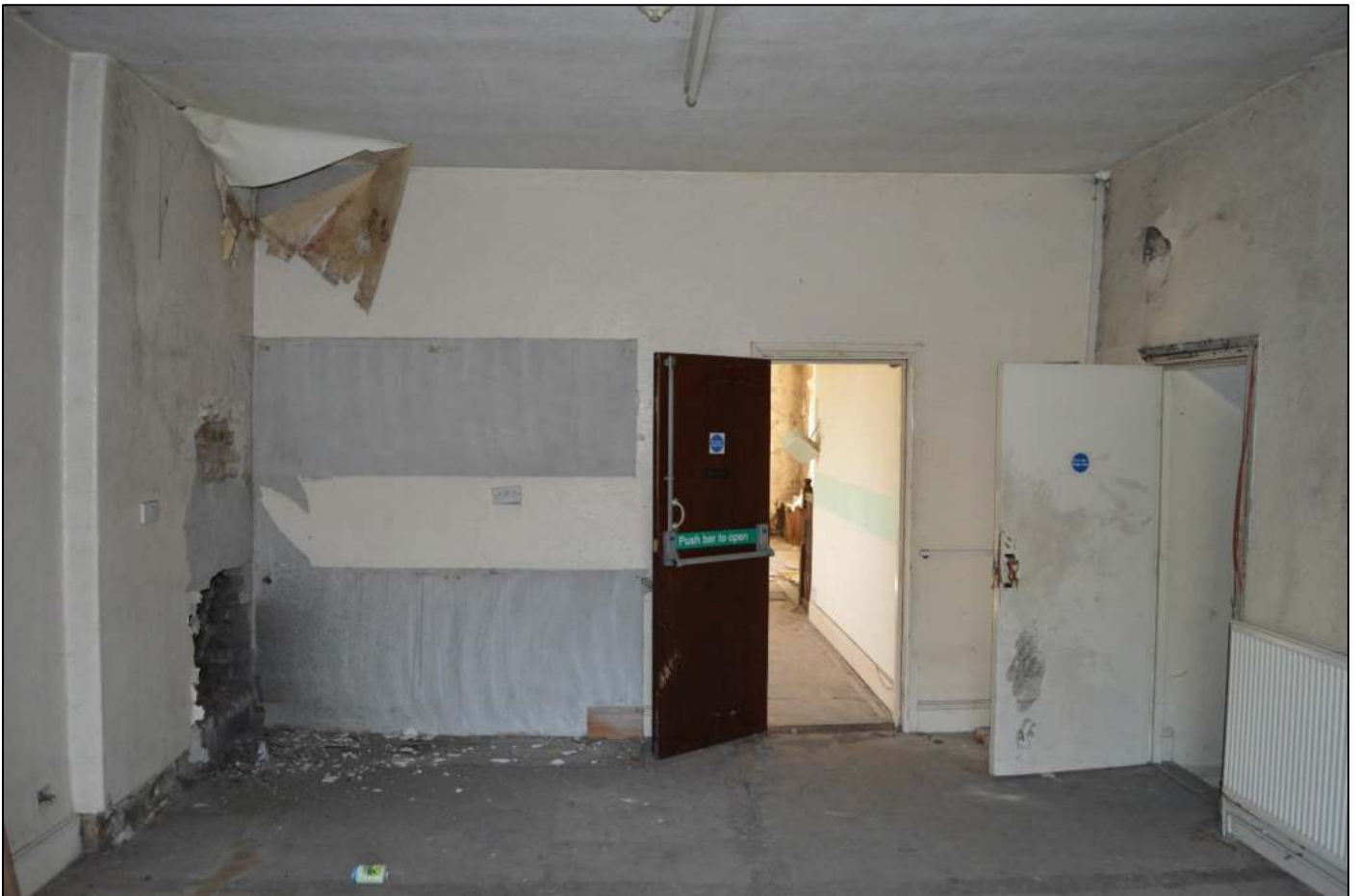
PL40: View south east within the rear first floor unit of the coach house addition.
