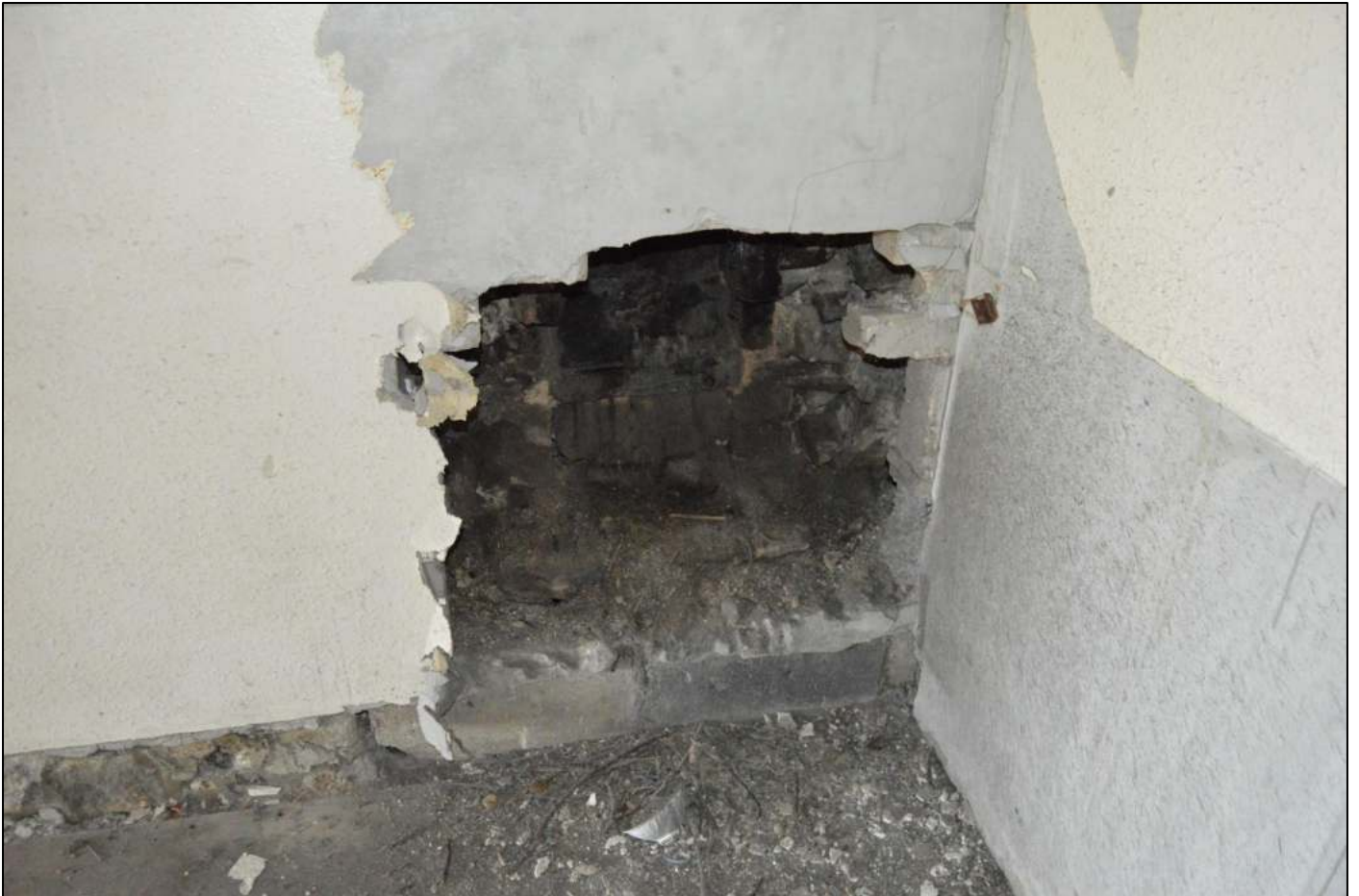
PL41: View of former fireplace opening to the chimney breast to the rear first floor unit of the coach house addition.
