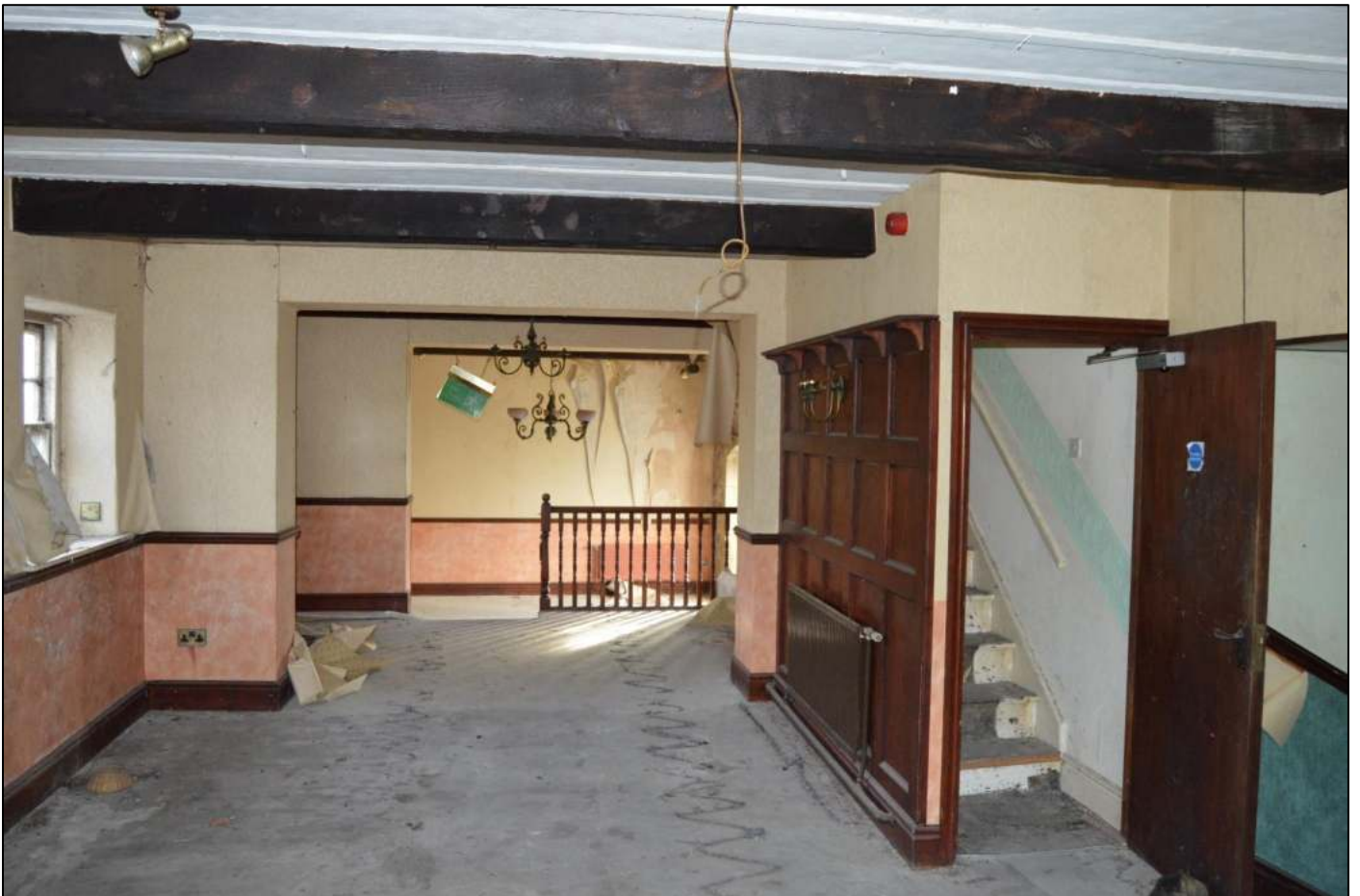
PL34: View north east within the rear ground floor unit of the coach house addition.
