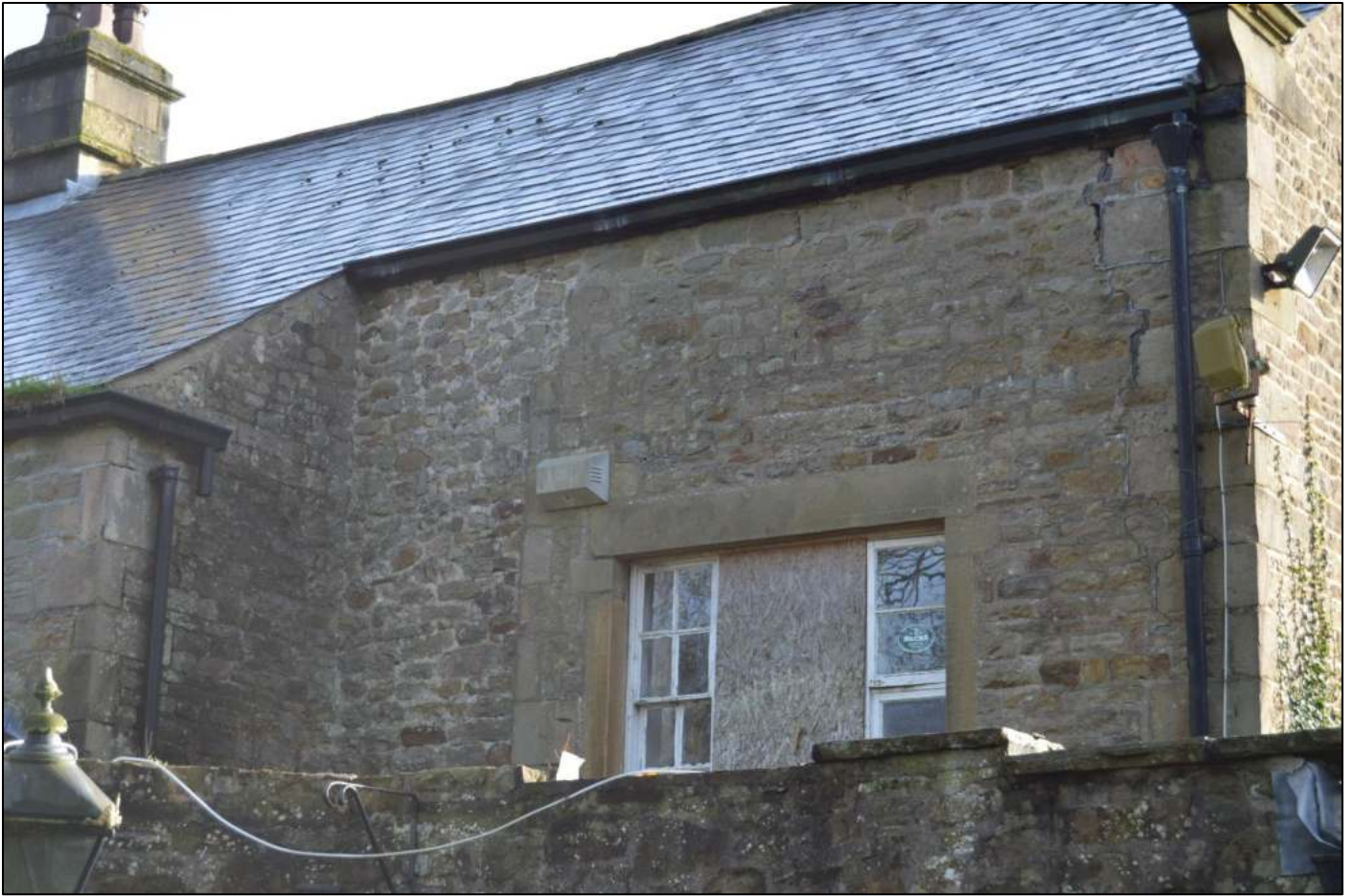
PL11: Evidence of alteration having occurred at first floor level to the south side of the rear north east elevation.
