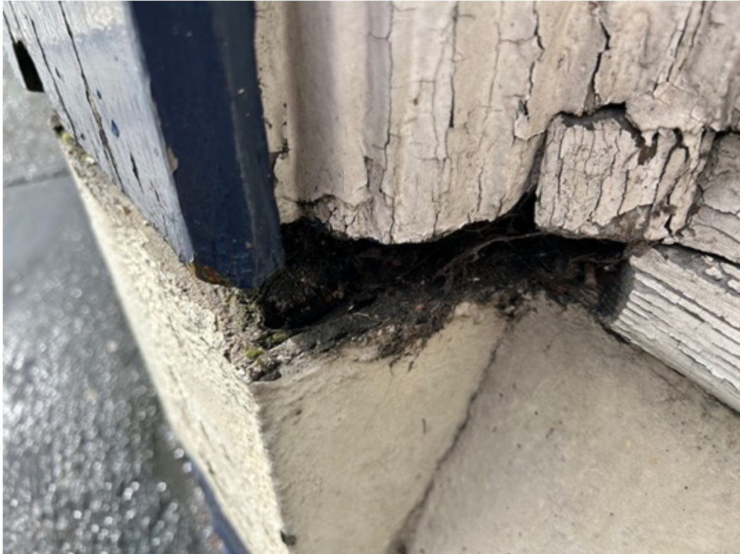
PL05: Junction between ground floor sash and pilaster. Render overlies timber forming the projecting pilaster detail.
