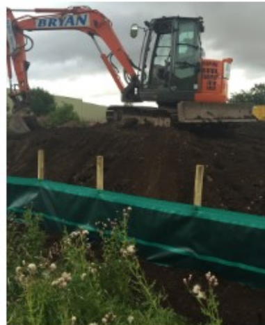
Silt Fence can be used as a temporary measure to prevent muddy water escaping from construction sites
