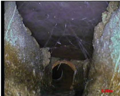
Observation [5]: INTERNAL MH
