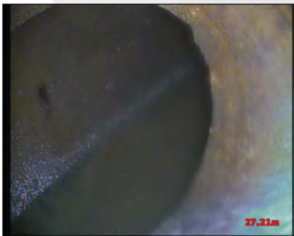
Observation [12]: MAIN DRAIN
