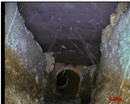
Observation [5]: INTERNAL MH
