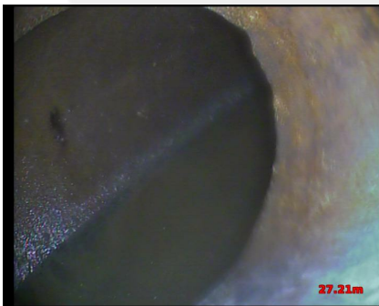
Observation [12]: MAIN DRAIN
