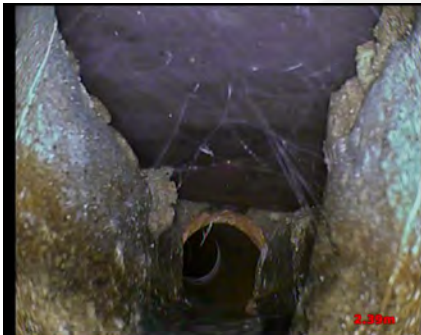
Observation [5]: INTERNAL MH
