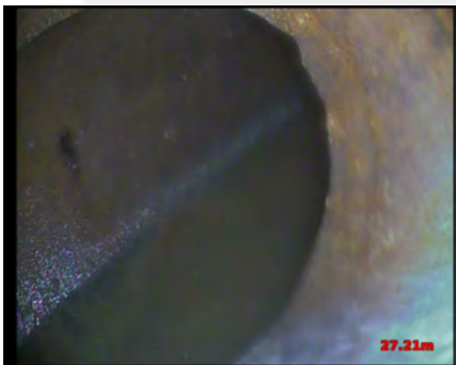
Observation [12]: MAIN DRAIN
