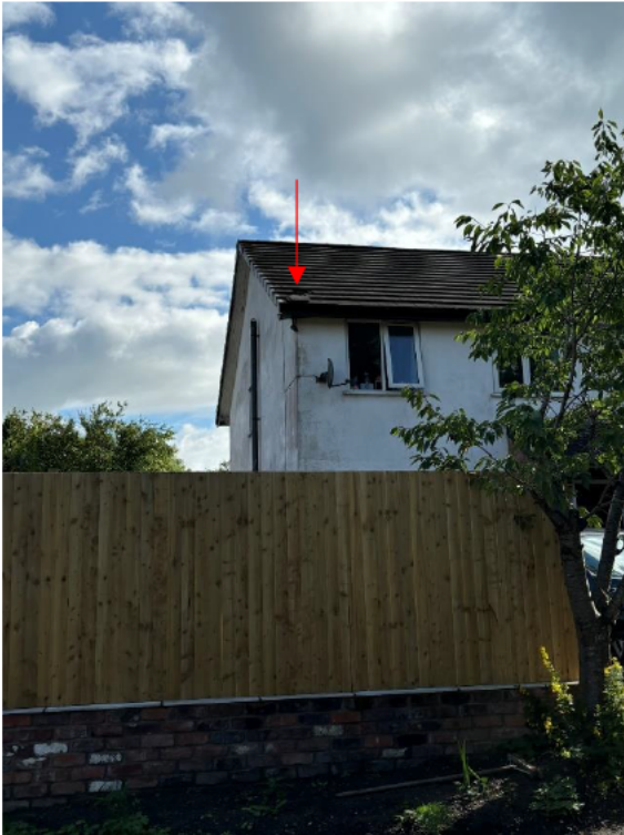
Photograph 1: Overview of the front elevation (southwest). Building in fair condition with missing roof tiles.
