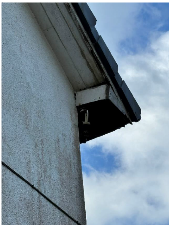
Photograph 6: View of the damaged wooden soffit on the west corner of the building. Wood appears water damaged.
