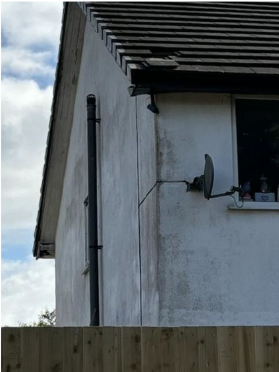
Photograph 2: Closer view of missing tile on southwest elevation. This has now been reinstated.
