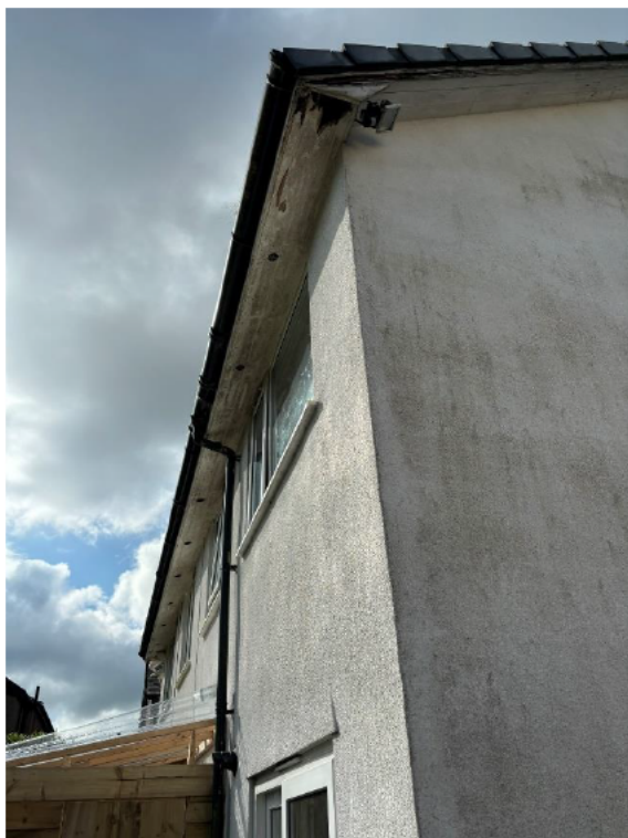
Photograph 5: View of the northeast (rear) elevation. Large hole in the wooden soffit board and visible damage further along soffit leading to northwest apex. Bird nesting.
