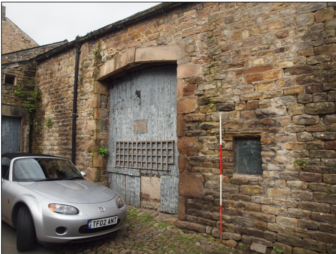
Plate 4: Barn door to have cill raised
