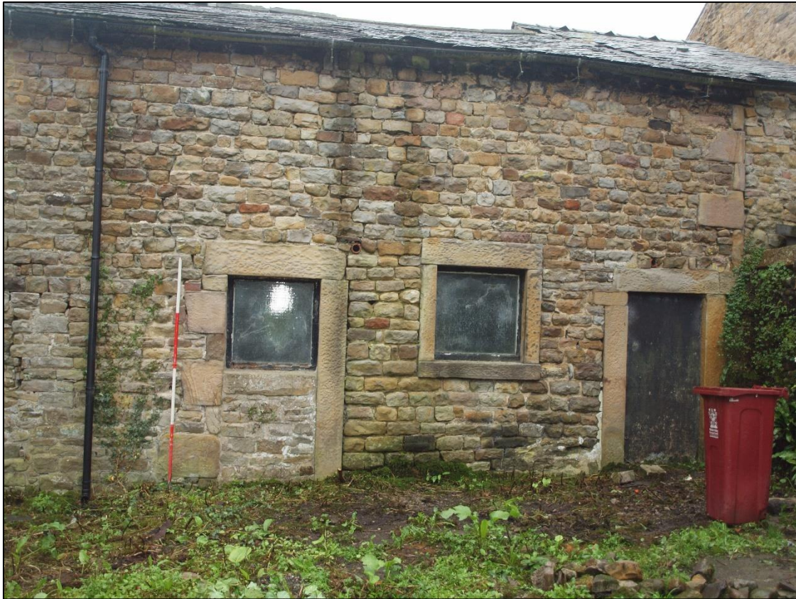
Plate 11: Doorways with cills and lintels to be raised and location of inserted first floor windows
