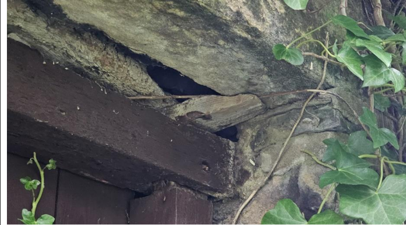
Photograph 10: Gap above doorway on substation which could be used by bats to access the building.
