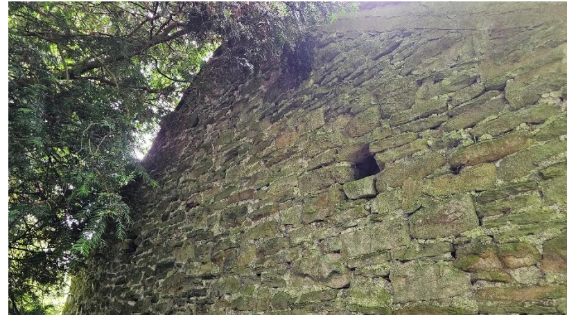
Photograph 8: Northern aspect of the substation, missing stonework/mortar provide numerous locations for roosting bats.
