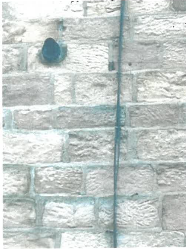
Close-up of Flue pipe emerging from the first floor bedroom cupboard.
