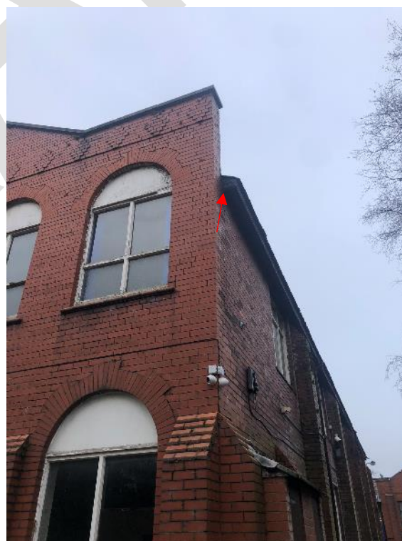
Photograph 4: Gap on south east corner where wooden soffit is damaged (PRF2).
