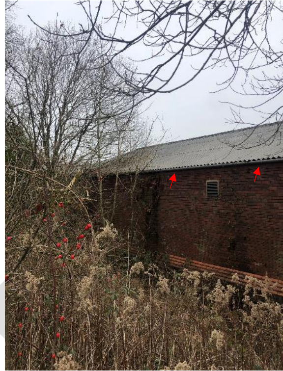
Photograph 11: Potential gap at top of wall due to absence of fascia board/soffit (PRF5). Unable to inspect closely due to watercourse.
