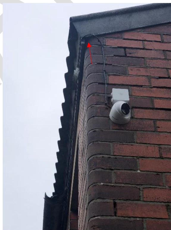
Photograph 8: Gap on north corner of building 2 behind asbestos fascia (PRF4).
