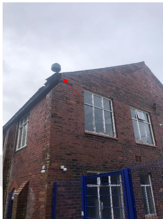
Photograph 3: Damaged wooden soffit allowing potential access to wall cavity (PRF2).
