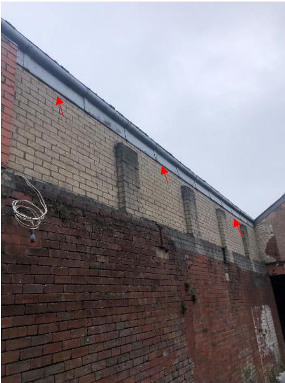
Photograph 10: Large overhanging asbestos fascia on west elevation of building 4 is off set from brick wall (PRF4).
