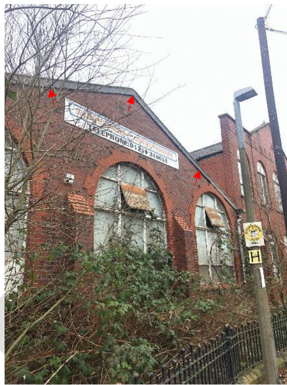
Photograph 7: Asbestos fascia on Building 2 is off set from the wall allowing access between wall and fascia board (PRF4).
