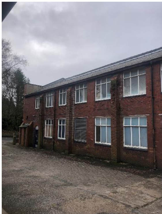
Photograph 1: View of the east elevation of Building 1. Gaps in roof slates and around skylight.
