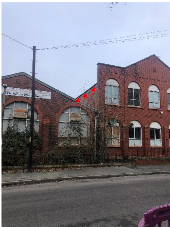
Photograph 5: Gap along western elevation of Building 1 where fascia board is missing (PRF3).
