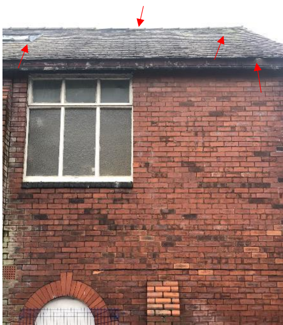
Photograph 2: View of the east elevation with dislodged slates and gaps around skylight (PRF1).
