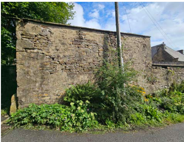
Figure 6 West facing elevation of the remains of the Heyhouses Cottages
