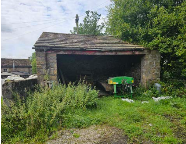
Figure 2 East facing elevation of the remains of the Heyhouses Cottages
