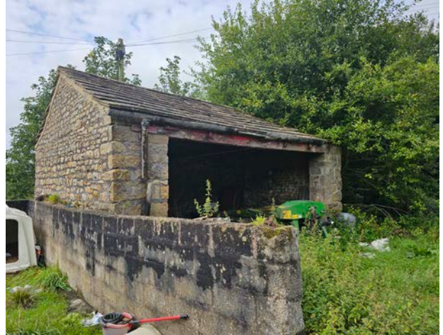
Figure 3 East facing elevation of the remains of the Heyhouses Cottages
