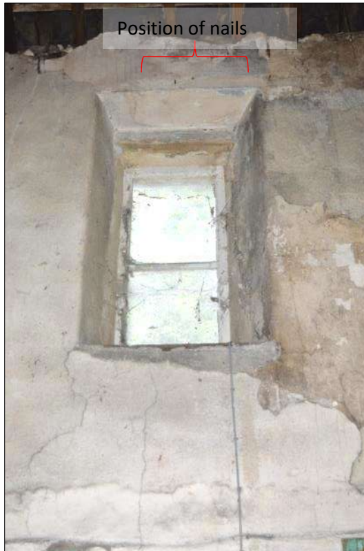
Plate 53 (shot 126): Close up of northwest first floor window with two protruding iron nails on the lintel, looking north-northwest
