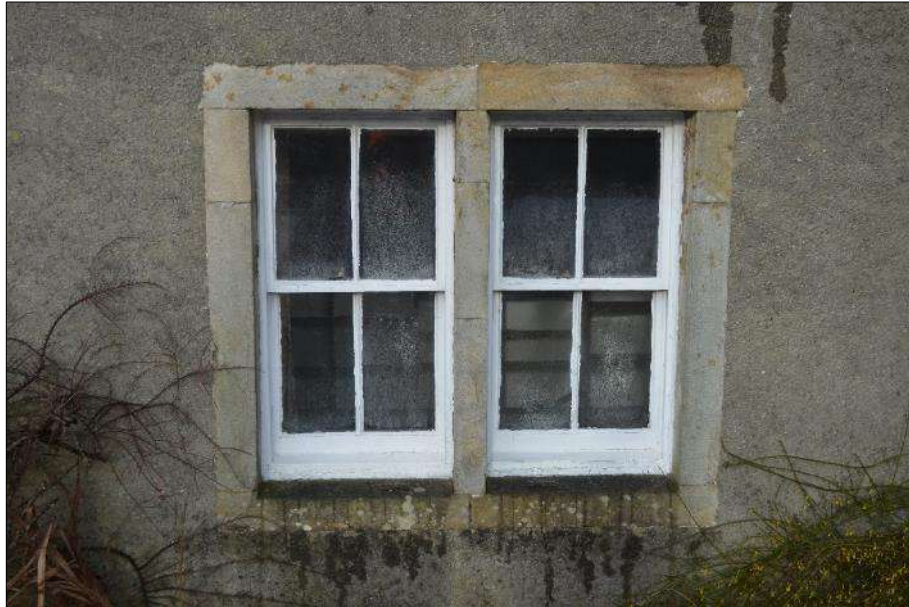
Plate 10 (shot 119): Close up of ground floor, recessed, sash window with glazing bars and no horn, looking north-northwest
