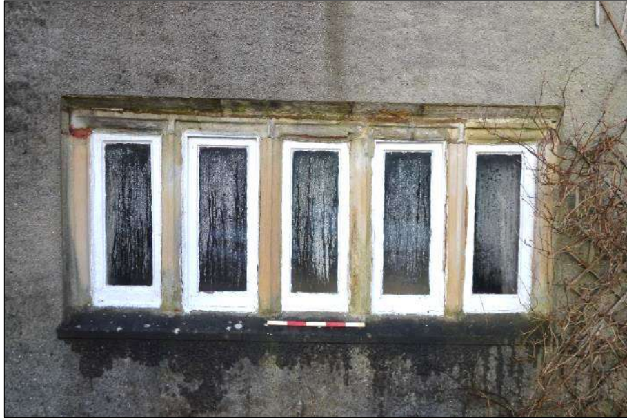
Plate 8 (shot 113): Mullioned 5-light window on the southeast elevation, looking north-northwest, 0.5m scale
