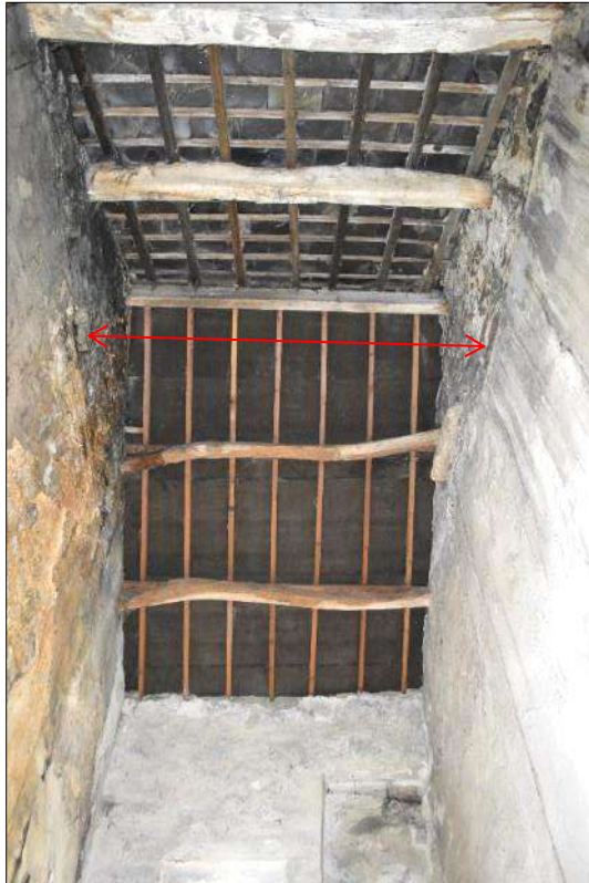
Plate 51 (shot 128): Purlin roof structure and niche or blocked opening on the southeast wall, first floor level, notice the lack of thick plaster on the gables, see arrow, looking southeast
