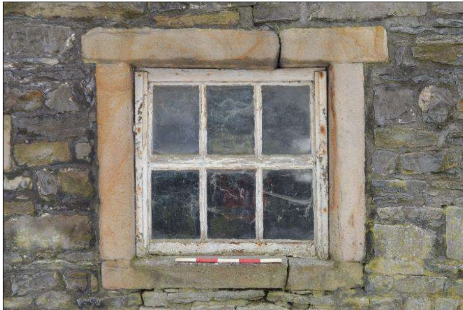
Plate 70 (shot 4): Timber window with top opening in with plain stone surround, looking southwest, 0.5m scale
