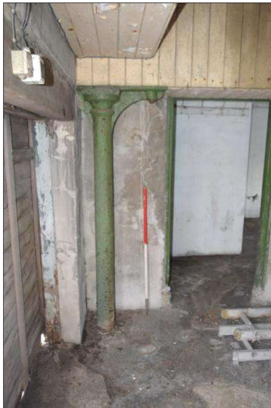
Plate 88 (shot 38): Close up of cast iron column along the northeast wall, looking southeast, 1m scale
