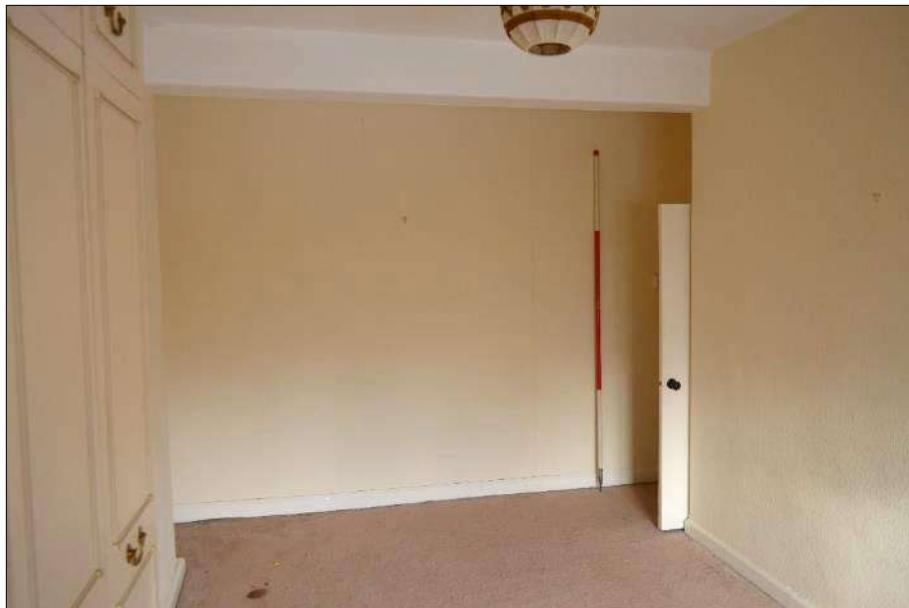
Plate 33 (shot 202): General view of bedroom (2.2) looking towards the staircase wall, looking north-northwest, 2m scale
