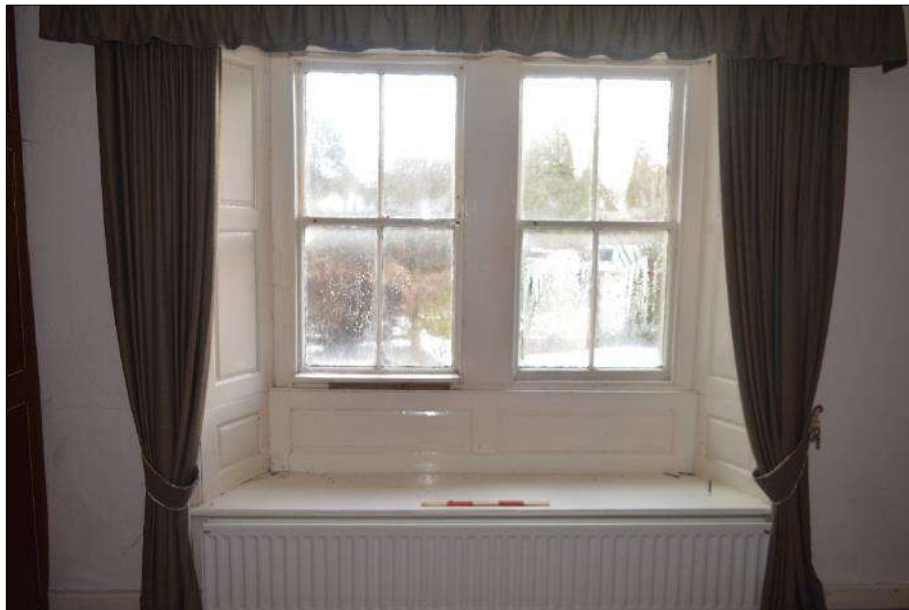
Plate 37 (shot 205): Close up of first floor bedroom window in (2.4), looking south-southeast, 0.5m scale
