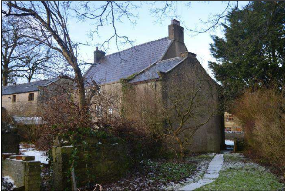
Plate 47 (shot 79): View of the extension (A2) and farmhouse (A2), notice the partially reduced chimneystack, looking northwest
