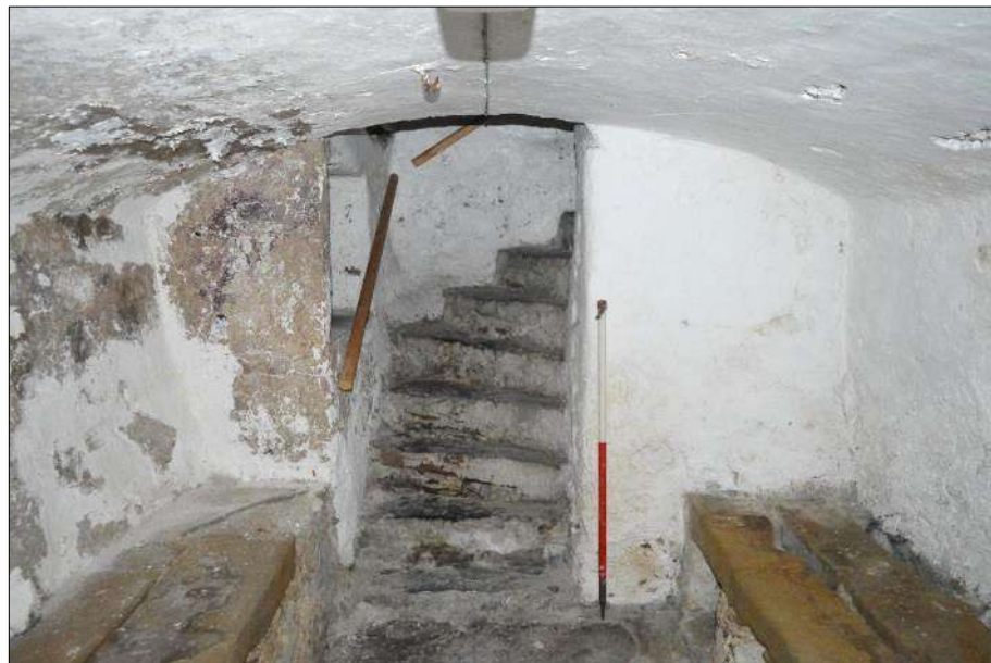
Plate 14 (shot 235): General view of the cellar towards the staircase, looking southwest, 1m scale
