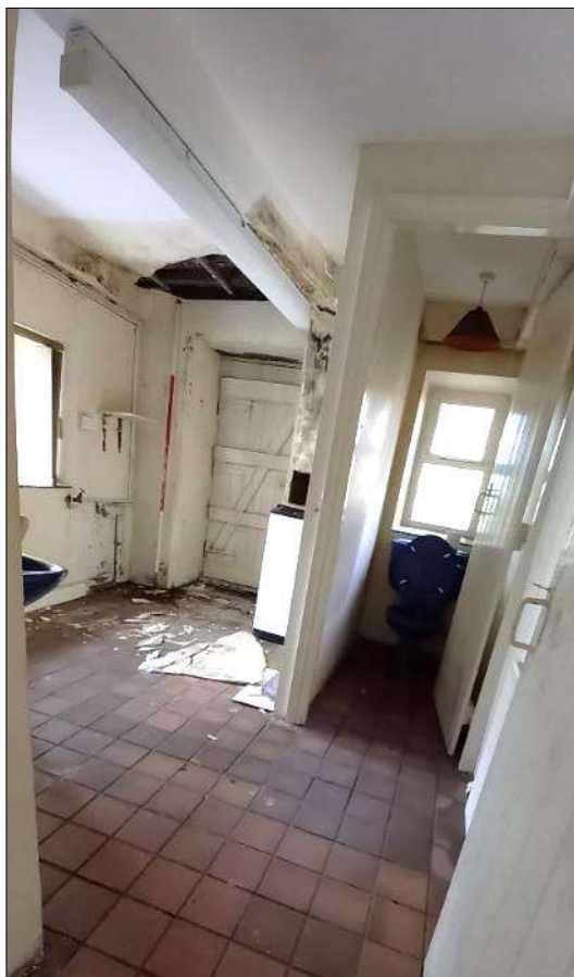
Plate 30 (shot 176): General view of the converted bathroom and WC, looking east-northeast, 2m scale
