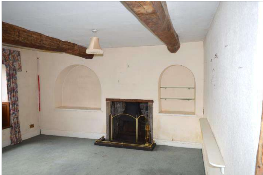
Plate 22 (shot 156): General view of the living room (1.2) towards the later wood burner and possibly later added niches, looking southwest, 2m scale
