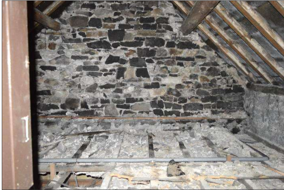
Plate 45 (shot 217): Roof space within the northwest wing, seen from room (3.1), looking north-northwest
