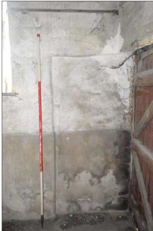
Plate 55 (shot 132): Recess to accommodate the door in the southeast wall, 2m scale
