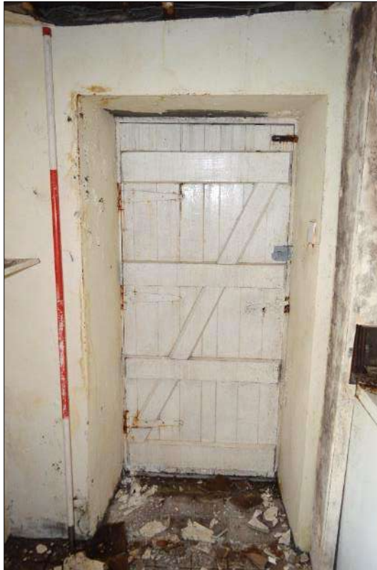
Plate 31 (shot 175): Plank and batten door with later brace, looking east-northeast, 2m scale
